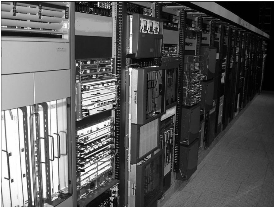
Figure 2-2 Rack-Mounted Network Equipment
