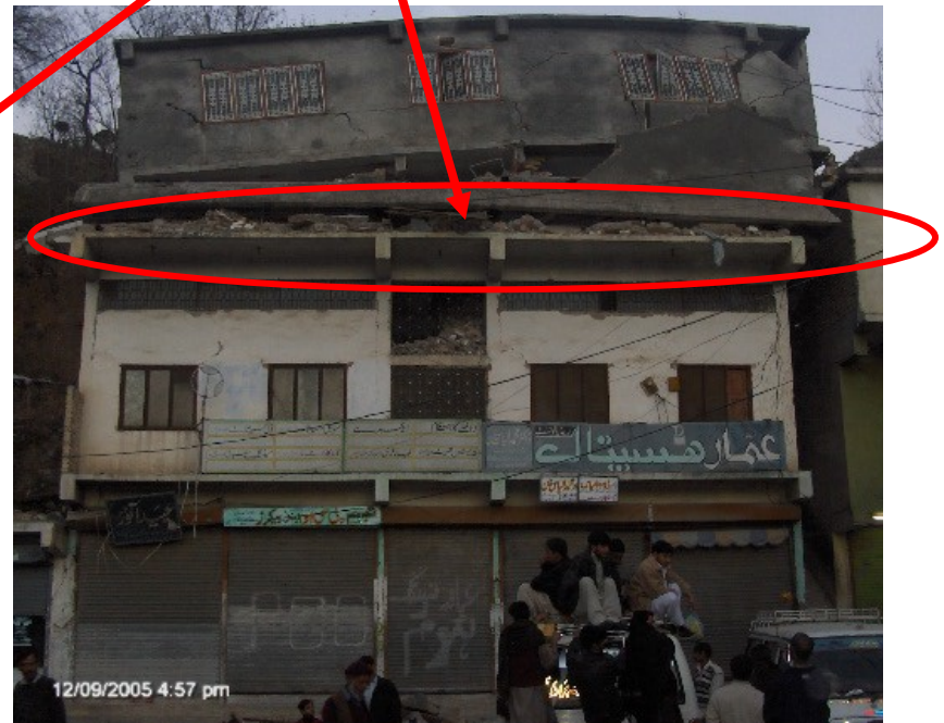
Bagh, 2005 Kashmir earthquake
