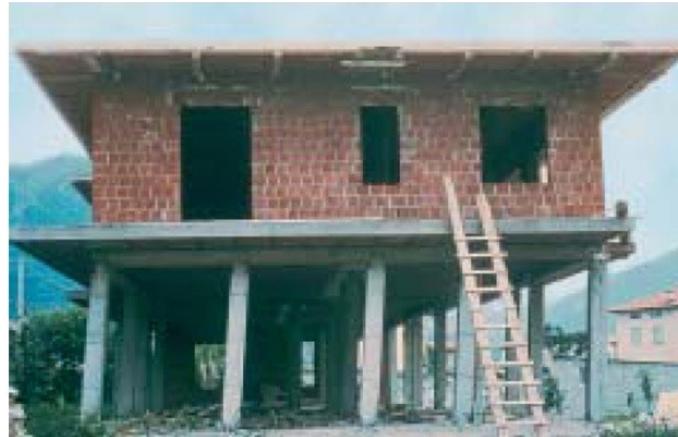
Permanent plastic deformation in the ground floor of a building under construction. Soft story effect almost provoked a collapse (Friaul, Italy 1976).
