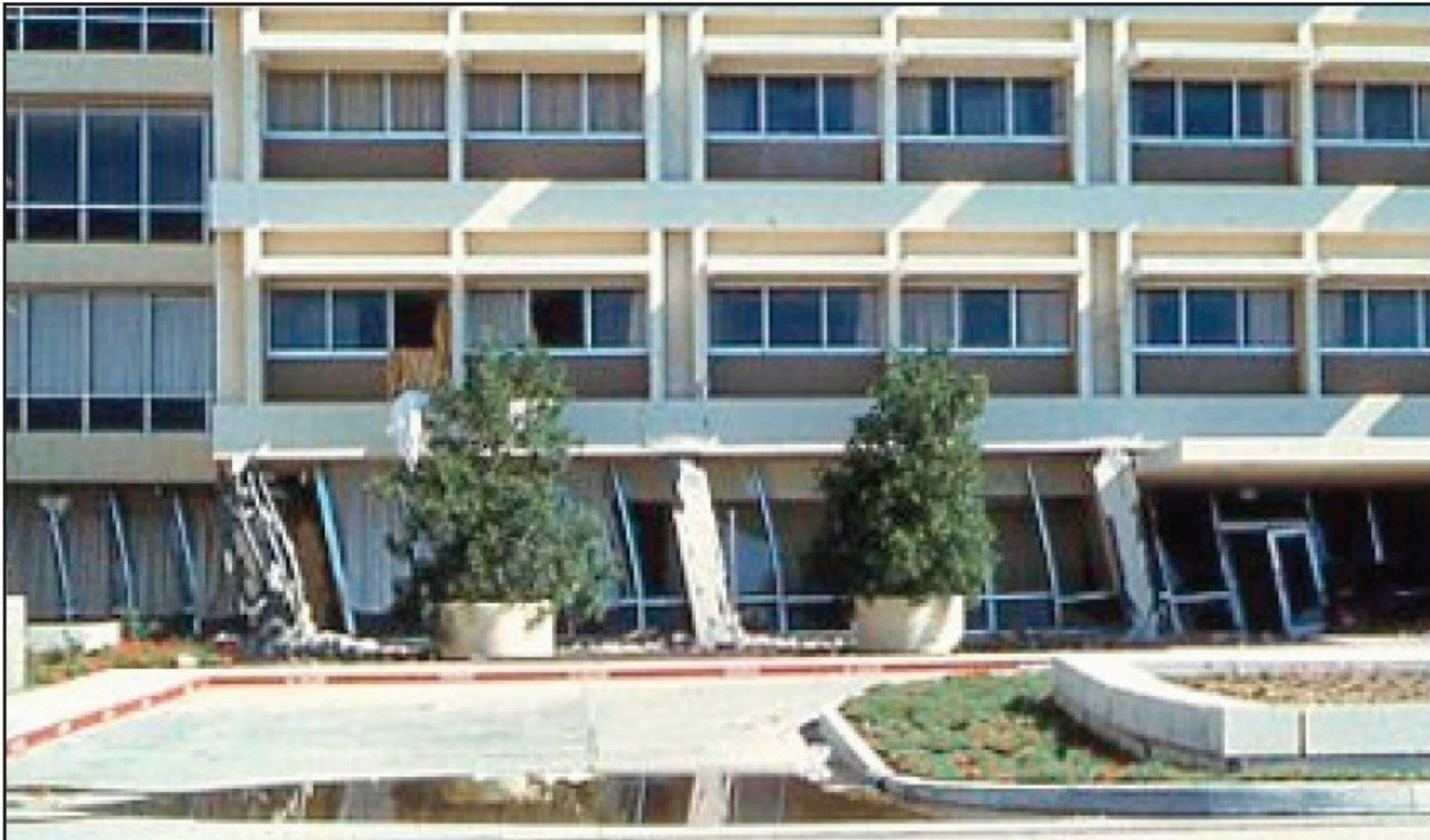
Olive View hospital, San Fernando earthquake, 1971, showing the extreme deformation of the columns above the plaza level.
