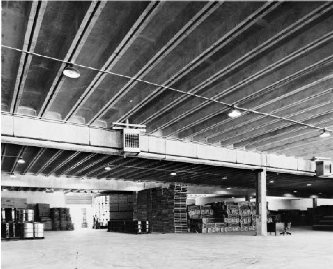
Prestressed concrete channels, John A. Denies Son Company Warehouse #4, Memphis, Tennessee. (Courtesy of Master Builders.)
