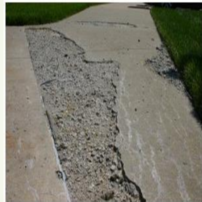
Pavement damage due to Freeze Thaw Cycles
