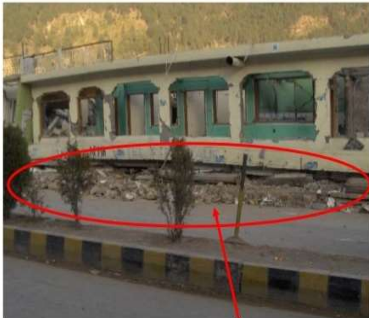
Lower story columns were collapsed in a hotel at Balakot, 2005 Kashmir earthquake
