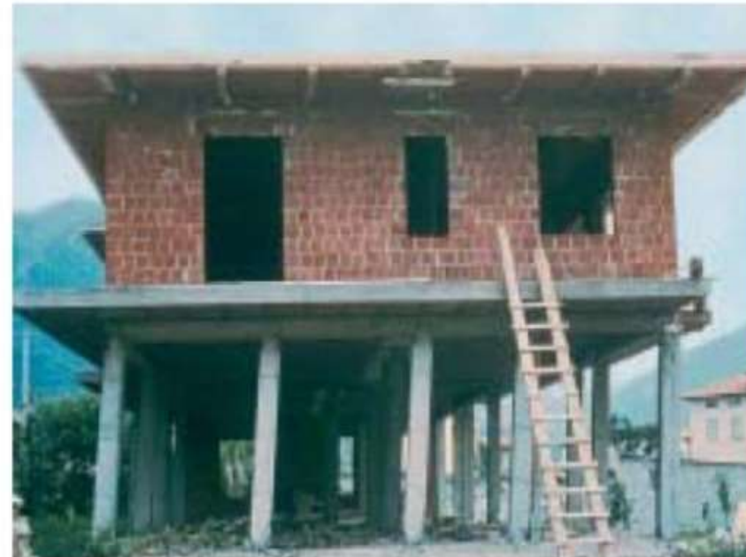
Permanent plastic deformation in the ground floor of a building under construction. Soft story effect almost provoked a collapse (Friaul, Italy 1976).
