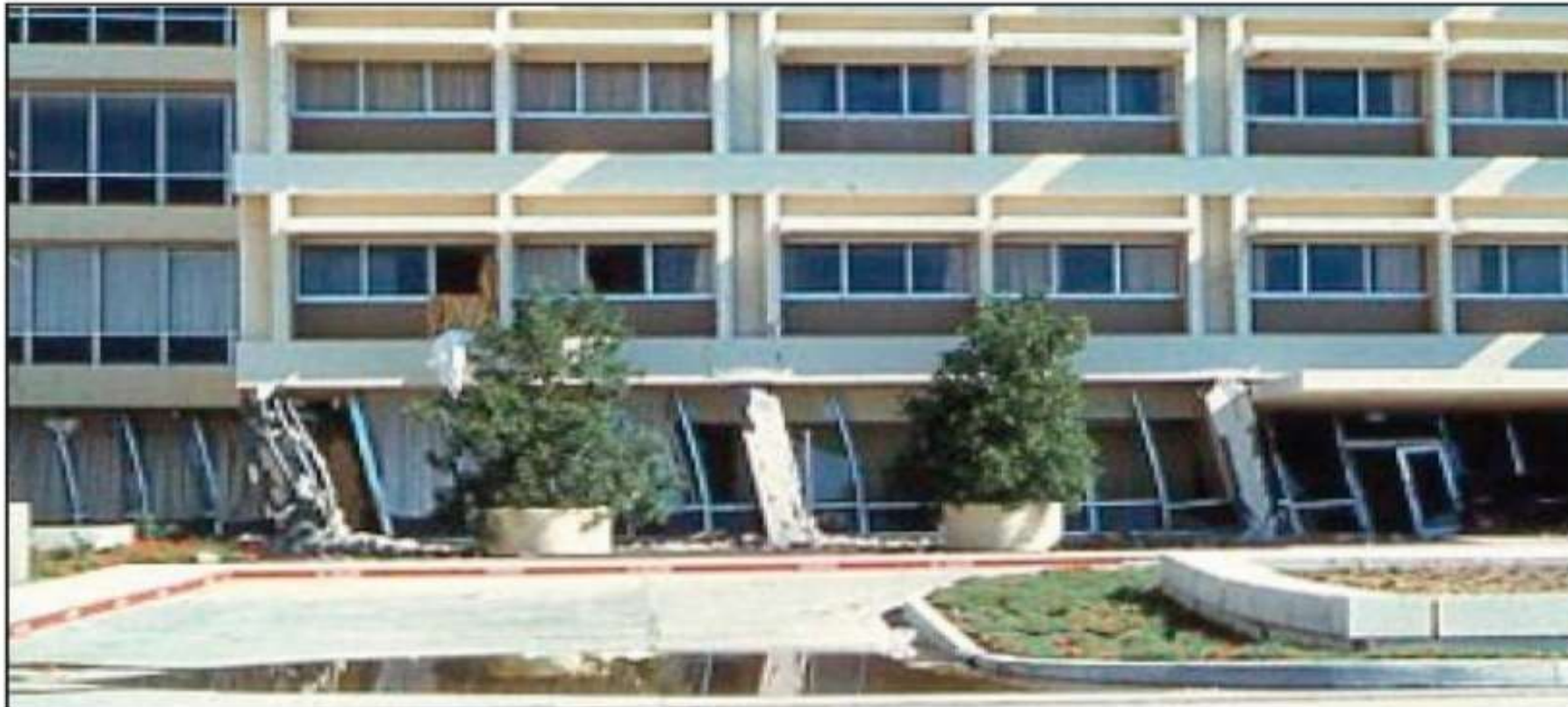
Olive View hospital, San Fernando earthquake, 1971, showing the extreme deformation of the columns above the plaza level.
