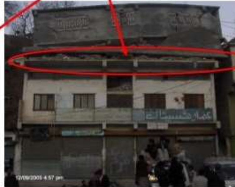
Bagh, 2005 Kashmir earthquake
