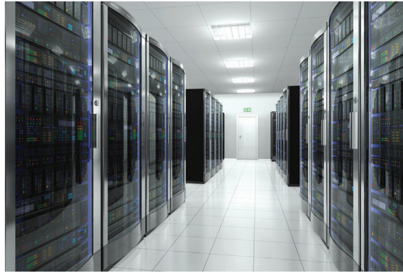
(b) A typical server room in a data center
