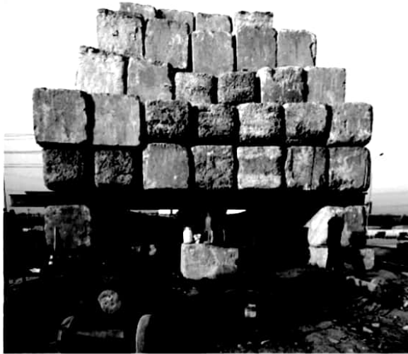
Figure 6: Pile Load Test platform with concrete blocks in pyramid configuration in Reach 3 (R3_PTP13)
