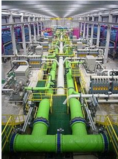
Reverse osmosis desalination plant in Barcelona, Spain
