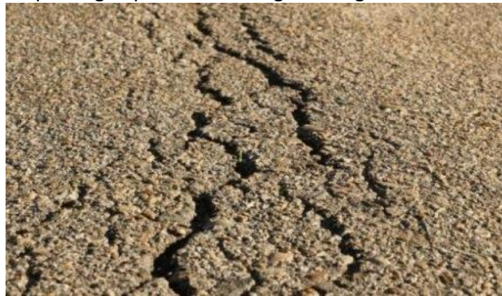
Fig 4: Shrinkage Cracks in Wet Compacted Soil
