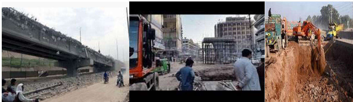
Fig 4: show the defective design of BRT
