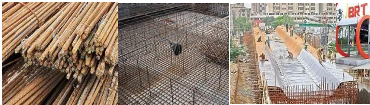
Fig 6: these picture are taken from sit of BRT project which show the corroded steal used in Project
