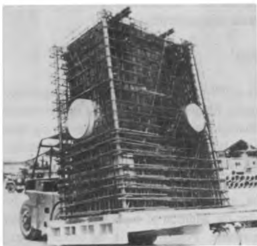
Figure 53. A general view of the high density steel reinforcement used in the voussoir elements.
