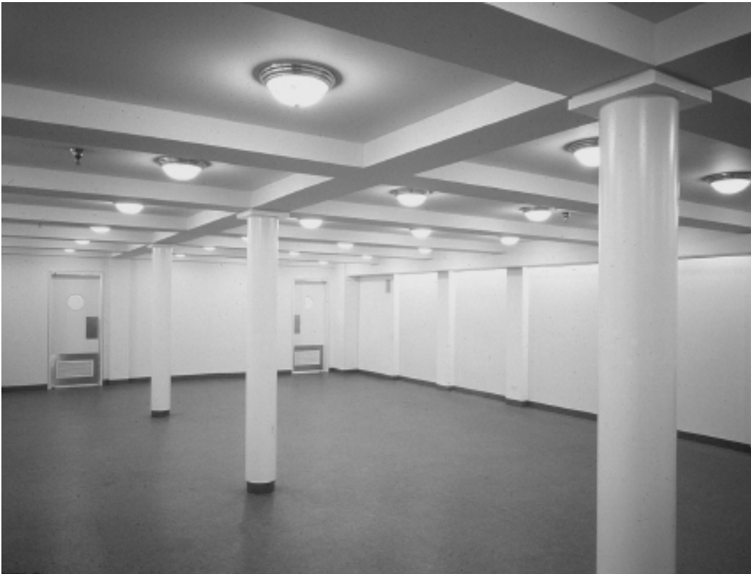
Figure 12.58 Ceiling-mounted diffuser luminaires.
