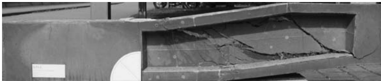
Fig. 5.15 Failure of fibre-reinforced UHPC beam without shear links [113]
