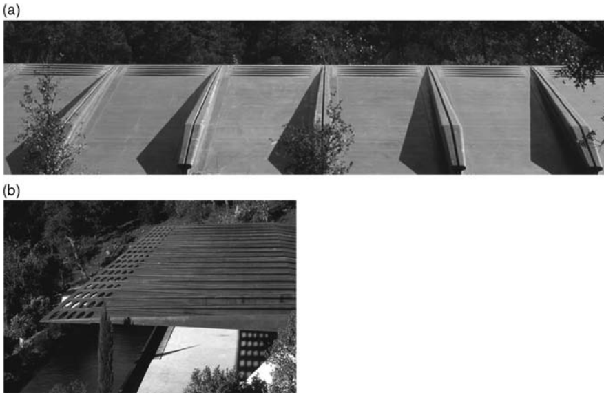
Fig. 7.59 Roof of precast UHPC segments at Villa Navarra, Le Muy, France [169]. a) several of the 17 identical, ribbed elements; b) cantilevering part
