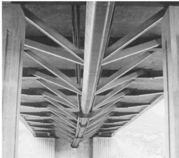
FIGURE 11.12 View of the Roize Bridge, France — space truss spans using tetrahedron modules.
