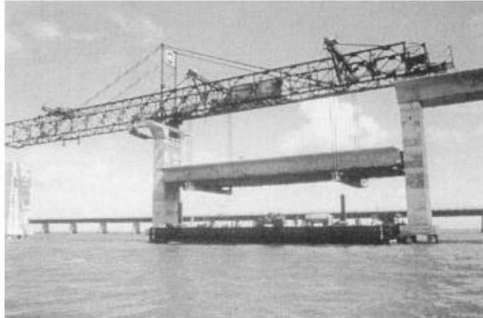
FIGURE 11.10 Lifting completed span of the Seven Mile Bridge, Florida, using an overhead truss .
