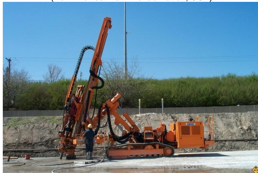
Fig. 7.13 – Grout holes are drilled at optimized angles for rock joints patterns (image from www.advancedconstructiontechniques.com/ ).
