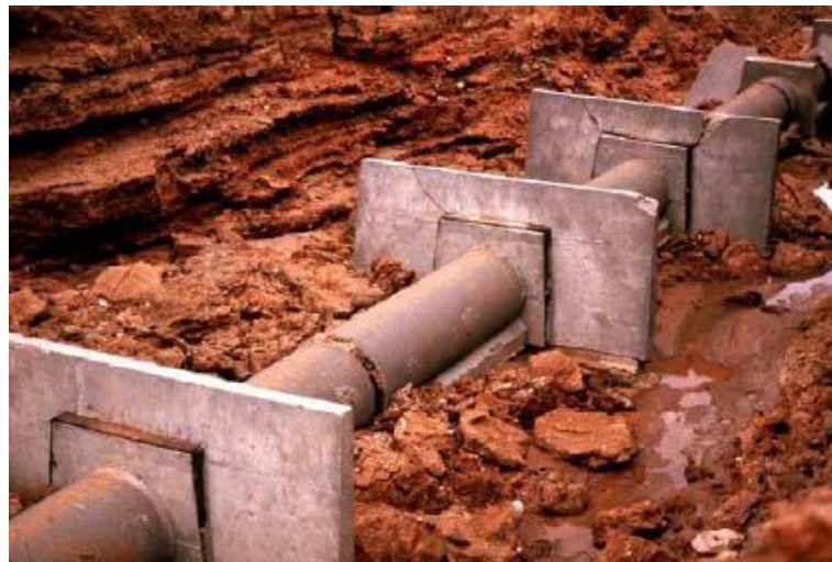
Fig. 5.6 – Pipe with intact anti-seepage collars shortly after failure of a small dam (McCook/2004).
