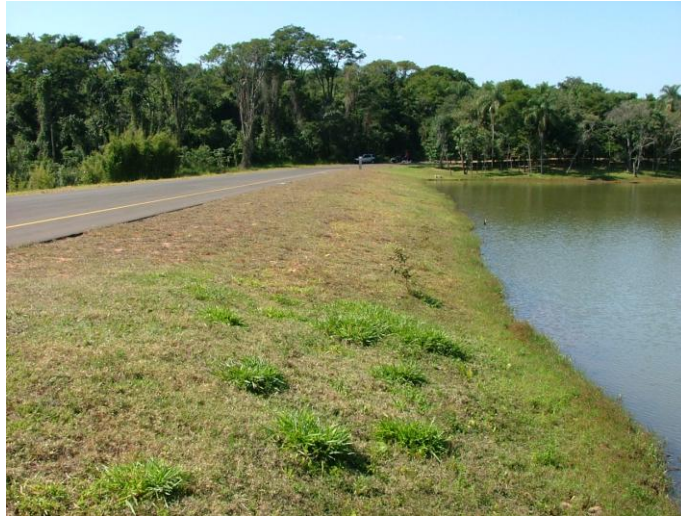
Fig.5.13 – Upstream slope protection with grass at the Chibarro dam, 12 m high, in Brazil (fetch = 300 m).
