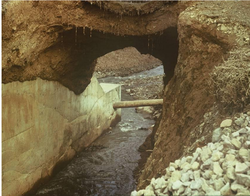
Fig. 3.8 – Earth Internal erosion after earth frost penetration along subtle spillway concrete wall
