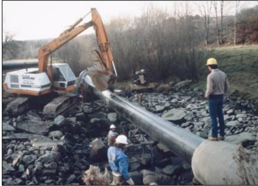
Fig. 7.16 – Example of sliplining – insertion of plastic (high density polyethylene) pipe into larger diameter concrete pipe (from FEMA, 2005)
