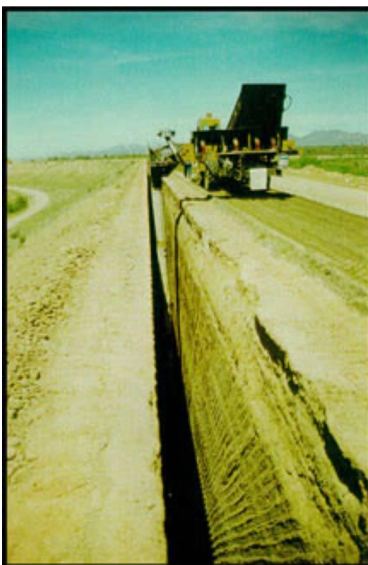
Fig. 7.14 – Central sand filter installed by open trenching from the crest of an existing low-height flood control dam in southwestern USA
