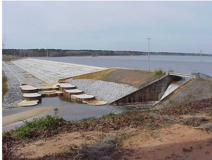
Fig. 7.8 – A view of principal and auxiliary spillways at Lake Tholocco Dam (Abdo and Adaska/07)
