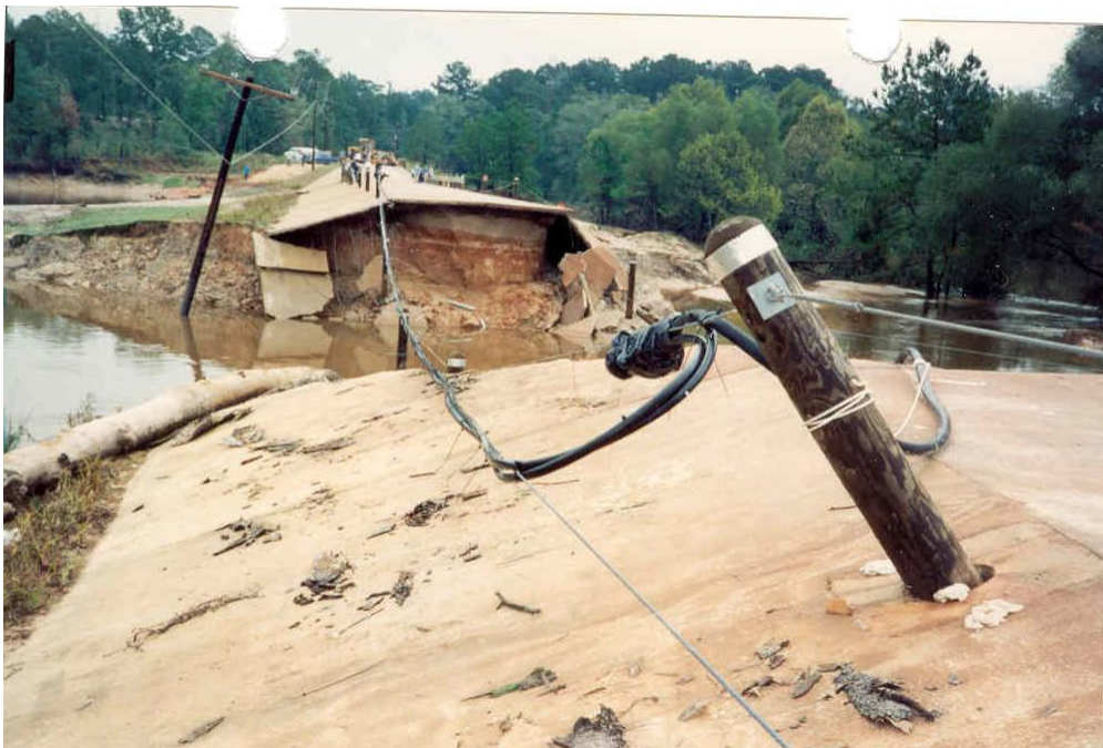
Fig. 3.5 – Consequences of the failure of Bear Foot Lake dam, in 1994 (ASDSO, 2007)
