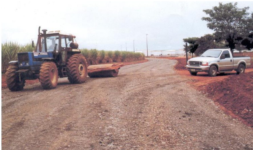
Figure 5.15 – Constructing a rural road using a granular material composed by gneiss, limestone and bituminous shale.
