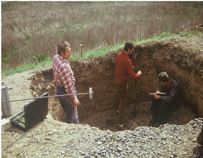
Fig. 3.7 – A sinkhole above failed bottom outlet concrete pipes, in a small dam.
