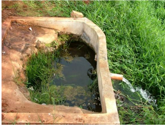
Fig. 6.3 – Vegetation debris upstream the weir gauge.
