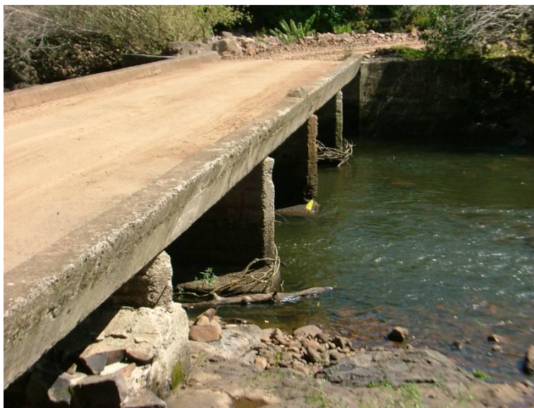
Fig. 8.3 – Type of bridge in the south of Brazil, with a resistant concrete structure, that is able to support high floods underwater.
