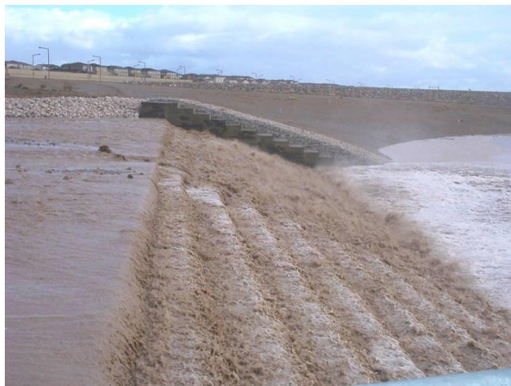
Fig. 7.10 – 2004 storm overview at Red Rock Detention Basin spillway (Abdo and Adaska, 2007)
