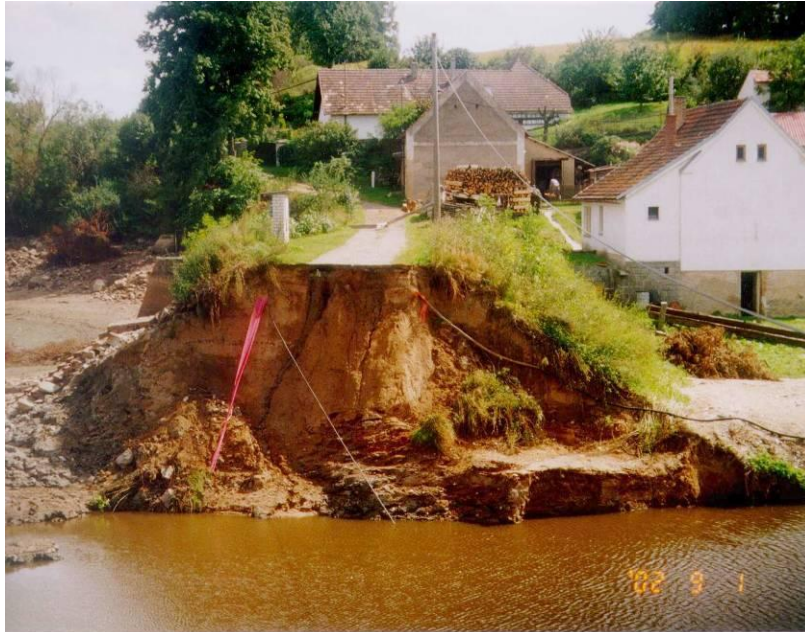
Fig. 3.2 – Massive dam break overtopping, during extremely high floods in the Czech Republic.
