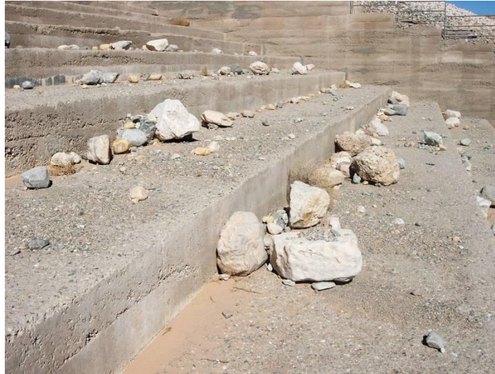
Fig. 7.11 – Boulders deposited on the RCC steps during 2005 storm (Abdo and Adaska, 2007)
