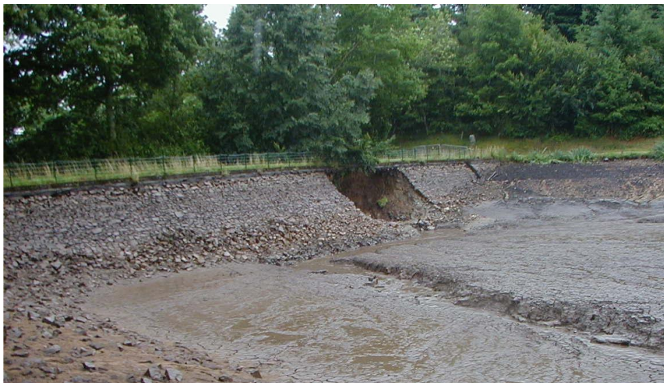
Fig.4.2 – France, Les Ouches small dam ( H = 5 \text{ m} , V = 49\,000 \text{ m}^3 ) collapsed by internal erosion in 2003, two centuries after completion [4].
