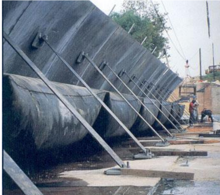
Fig.2.19 – Spillway gates with inflatable air bladders
