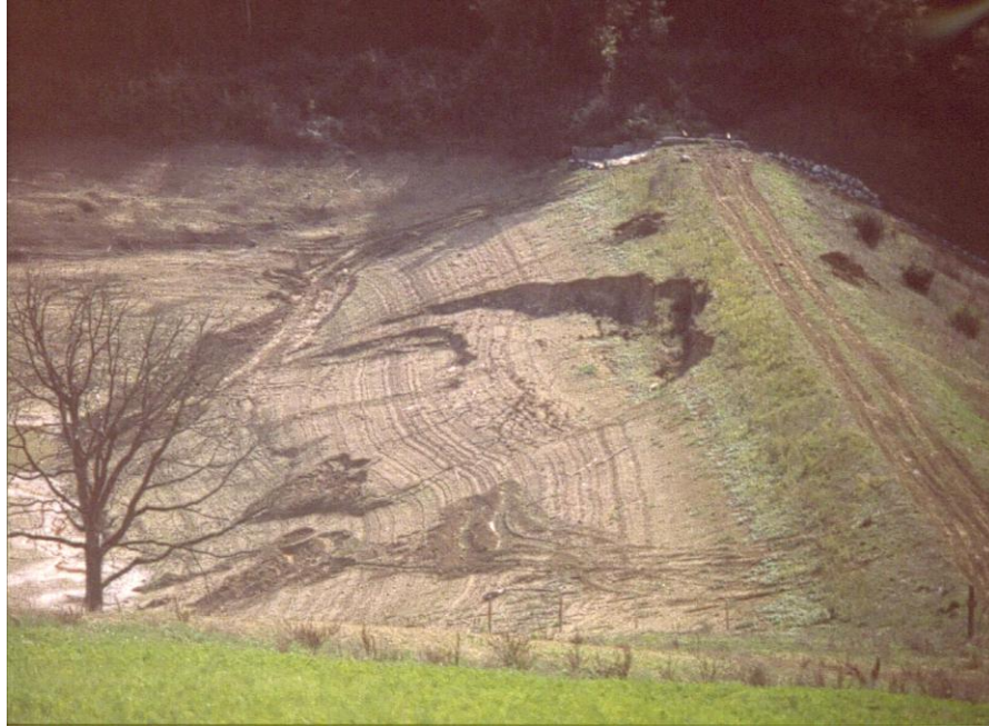
Fig. 3.10 – Sliding of upstream slope of a homogeneous embankment dam after rapid drawdown (France)
