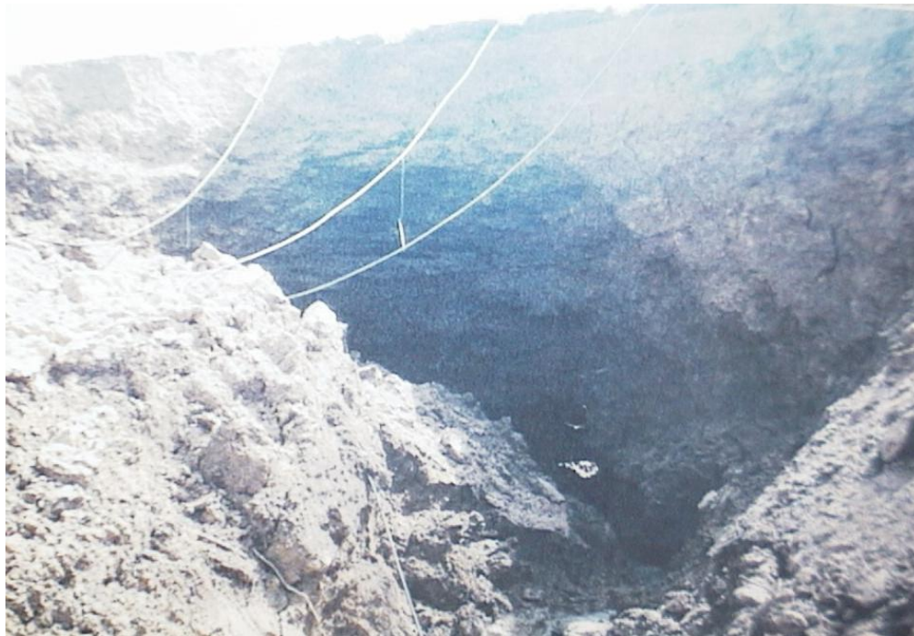
Fig. 3.9 - Pipe developed due action of water on dispersive soils (South Africa)
