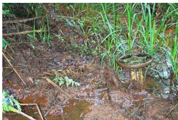
Fig. 7.19 – What are the chances that this valve will work in an emergency? (SMEC/2006)
