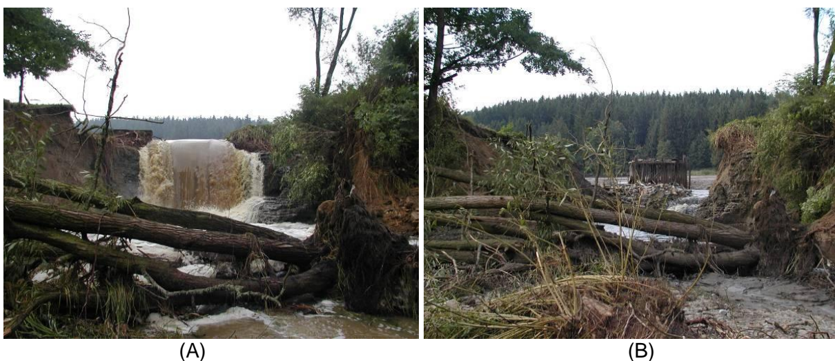
Fig. 3.1 – A small dam during the overtopping (A) and after the failure(B). (Czech Republic).
