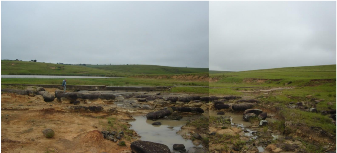
Fig. 7.1 – Backward erosion of the by-wash Spillway of Toleni Dam in South Africa
