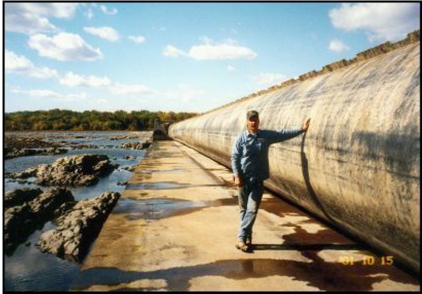
Fig. 2.18 – Photo of an inflatable dam at Sunbury, PA, USA [3]
