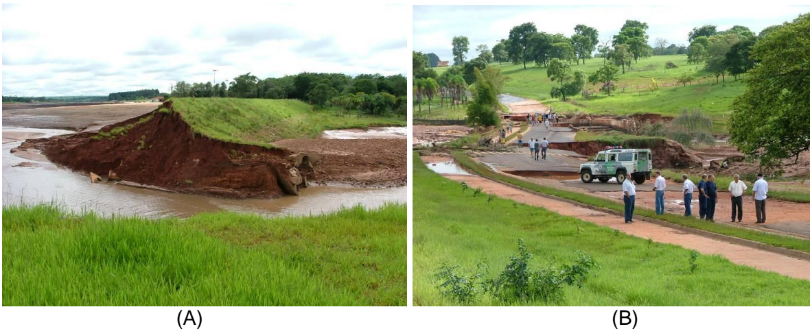
Fig. 3.3 – (A) Paraguaçu embankment dam failure by overtopping, after severe flooding in Brazil. (B) Downstream erosion damages at an embankment road access, in January, 2007.
