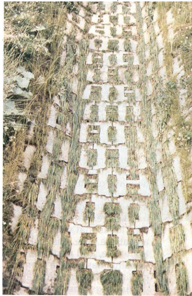
Fig. 7.6 – One of the cable-stayed block systems remains totally intact after a water test
