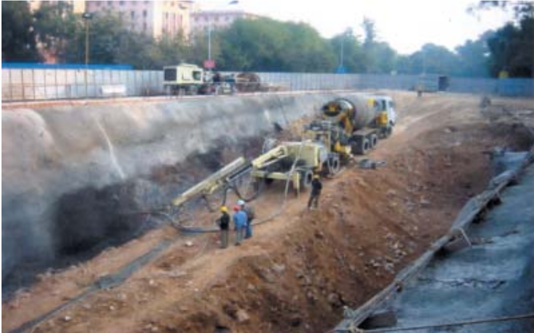
Shotcreting for slope protection by Robot Jet Machine at central secretariat, Delhi Metro.
