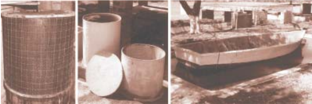
Small diameter wires and chickenwire mesh reinforcement used in casting ferrocement water tank
