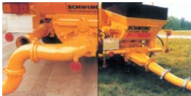
Pump and pipeline
