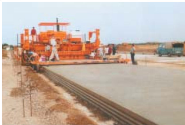
Paving concrete by slip-forming to get sinusoidal profile for linking with the adjacent slab.
