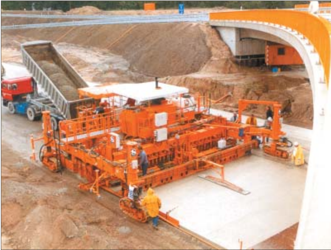
Placing high quality concrete by slip-form technique for a width of 8.5 m.
