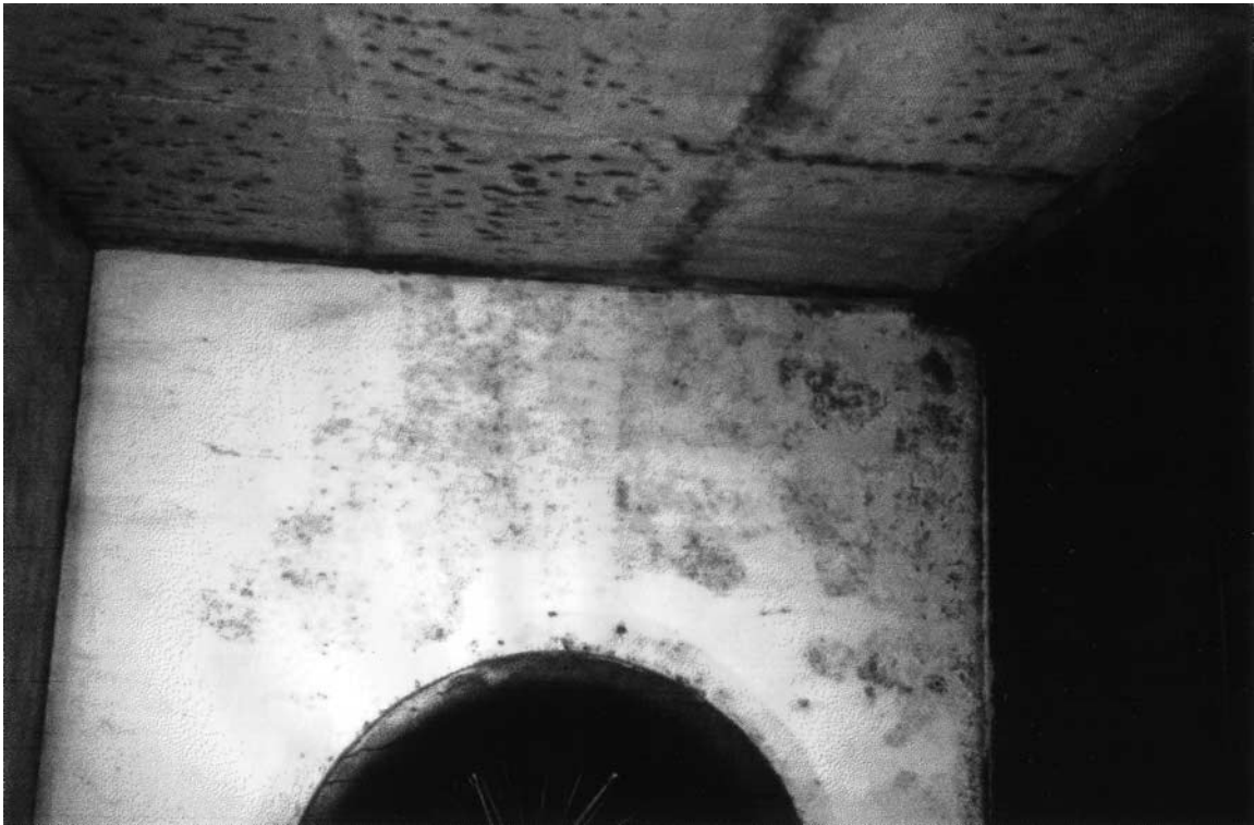
FIG. A-54 Corrosion in plenum. (Source: Altair Filters International Limited.)
