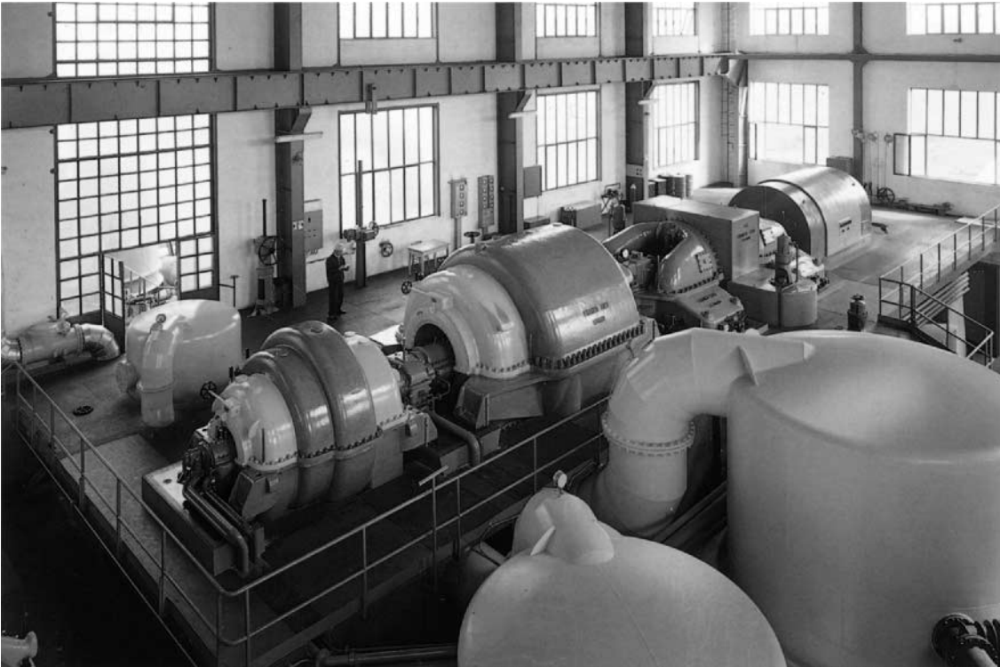
FIG. E-44 Compressor set for Castelnuovo geothermal power plant (Italy). (Source: Ansaldo.)
