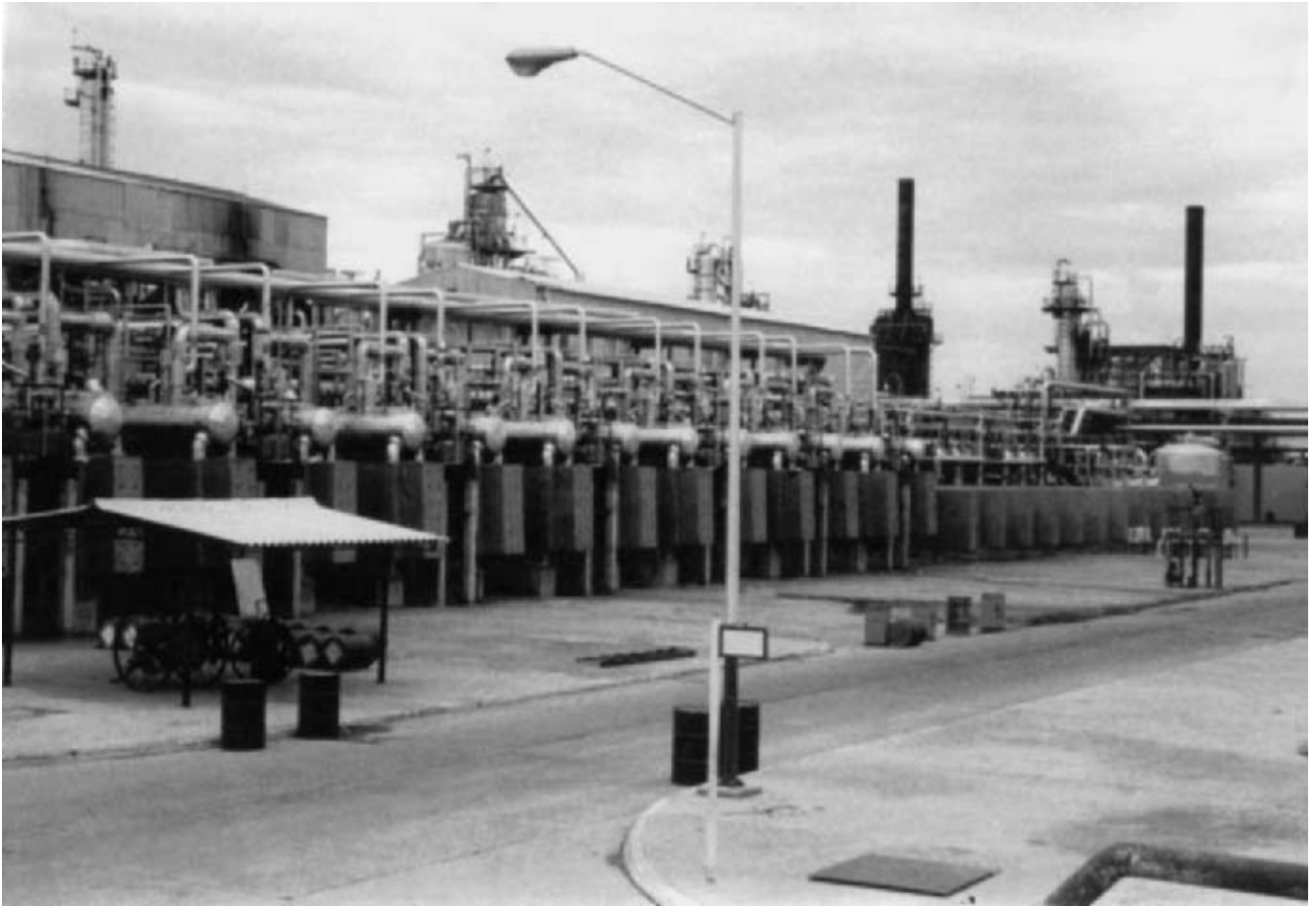
FIG. C-47 Large installation of wax crystallizers in a petroleum refinery. (Source: Armstrong Engineering Associates.)
