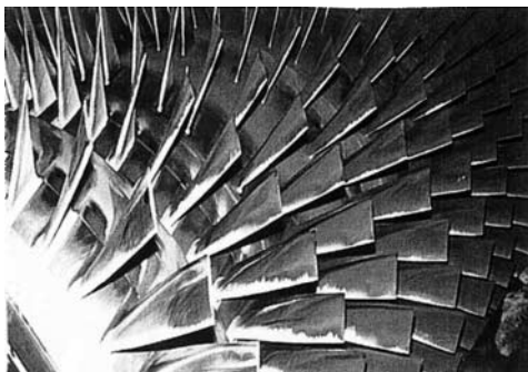
FIG. T-57 Picture of a compressor that was washed online every four days with detergent during approximately a one-month continuous operation period. (Source: Stalder.)
