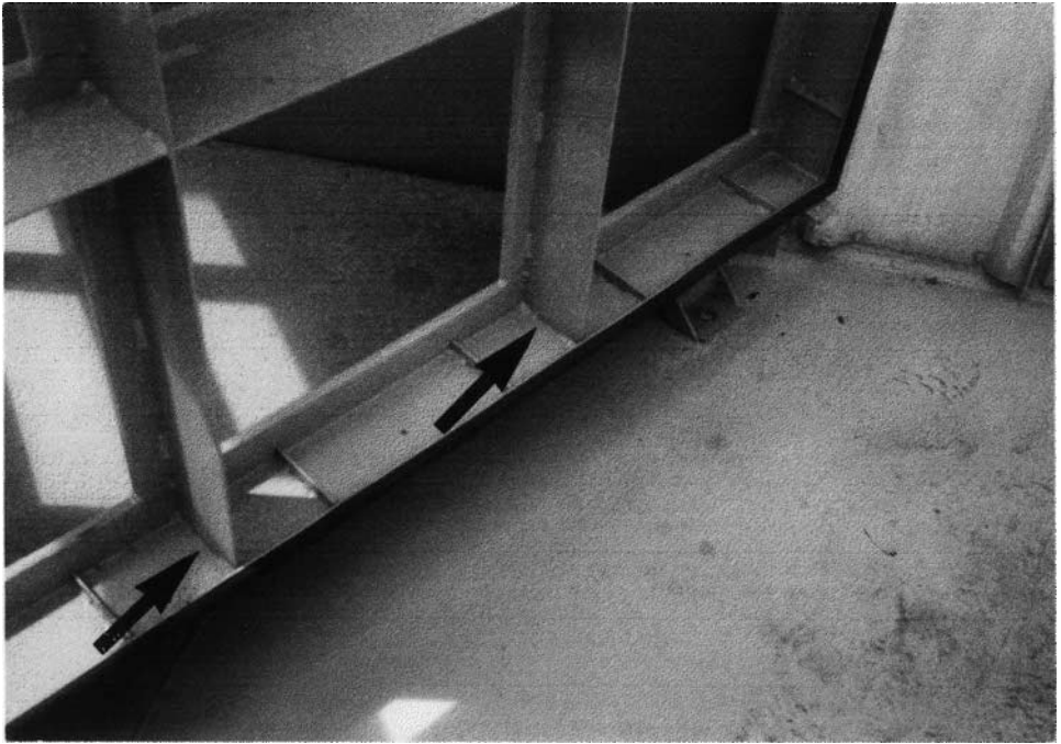
FIG. A-63 Corrosion on the new housing shown in FIG. A-62. (Source: Altair Filters International Limited.)
