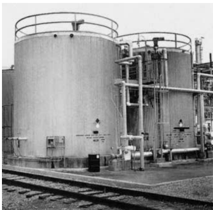
FIG. C-39 Typical TDI storage tank. (Source: ARCO Chemical.)
