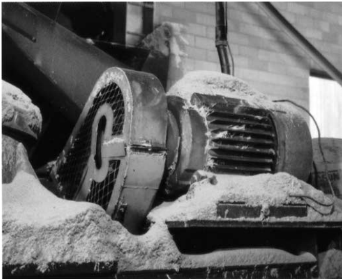
FIG. E-20 Motor-driven paper mill waste handling conveyor. (Source: Reliance Electric.)
