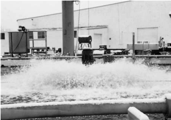
FIG. E-22 Motor-driven aeration pumps in secondary sewage treatment operation. (Source: Reliance Electric.)
