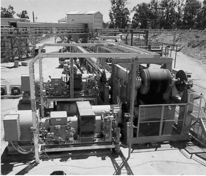
FIG. B-36 VHBI 316 with stepup gear, flange-mounted to a reduction gear in one of the drive stations in a 10-km-long conveyor plant, made up of several conveyor belts, for the conveyance of bauxite in West Australia. (Source: J.M. Voith GmbH.)
