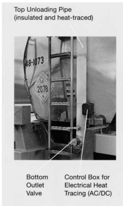
FIG. C-34 Tank truck unloading. (Source: ARCO Chemical.)
