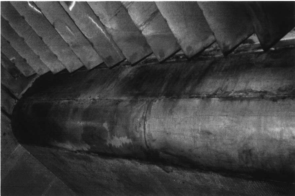
FIG. A-52 Corrosion at silencer outlet. (Source: Altair Filters International Limited.)
