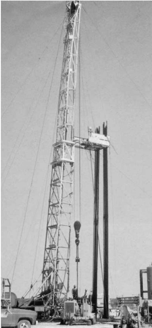
FIG. B-30 VHBI 422 D, fitted in the drive to the winch of a transportable drilling rig suitable for drilling to a depth of approximately 5000 meters, Texas, USA. (Source: J.M. Voith GmbH.)
