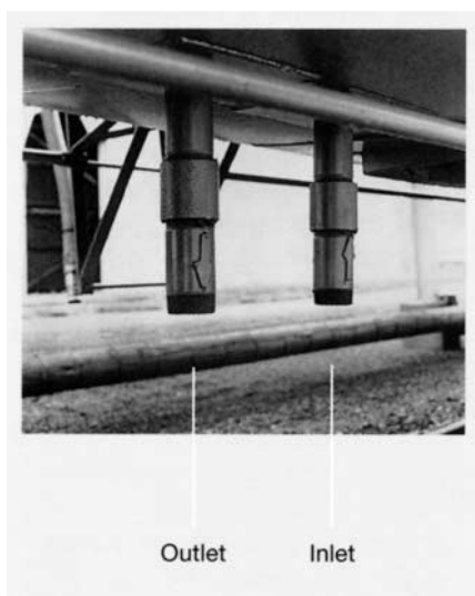
FIG. C-38 Steam hose connections. (Source: ARCO Chemical.)
