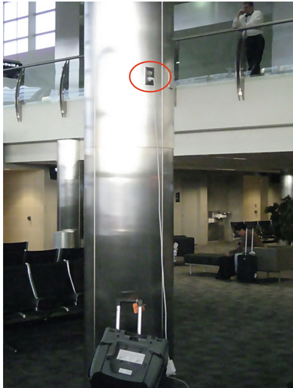
Fig. 12.3 An electrical outlet ( circled ) on a column designed to be difficult to use?
