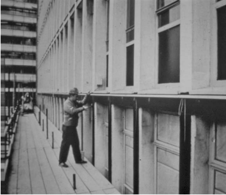
Fig. 11.9 A conductive paint coating applied to a building suffering from calcium chloride admixed into the concrete on the lowest two floors during construction. (Courtesy of Taylor Woodrow Construction)
