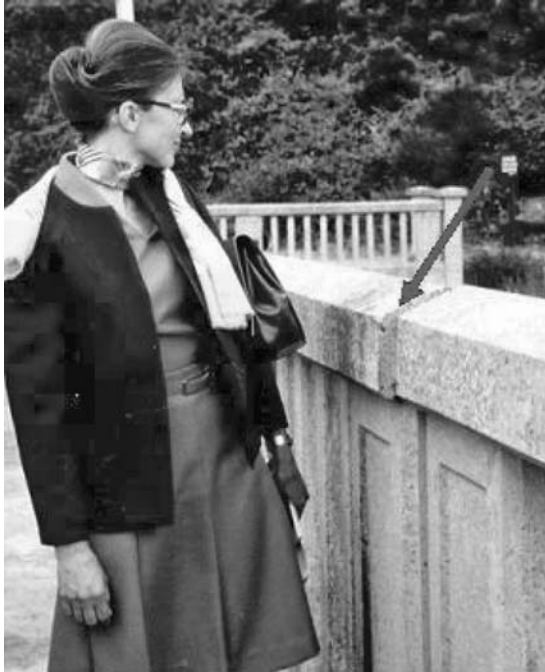
Fig. 4.10 A 50mm displacement upstream (arrowed) of the bay nearest the camera: Val de la Mare Dam, Jersey. (Reproduced with permission from Poole. 68 © Alan Poole)
