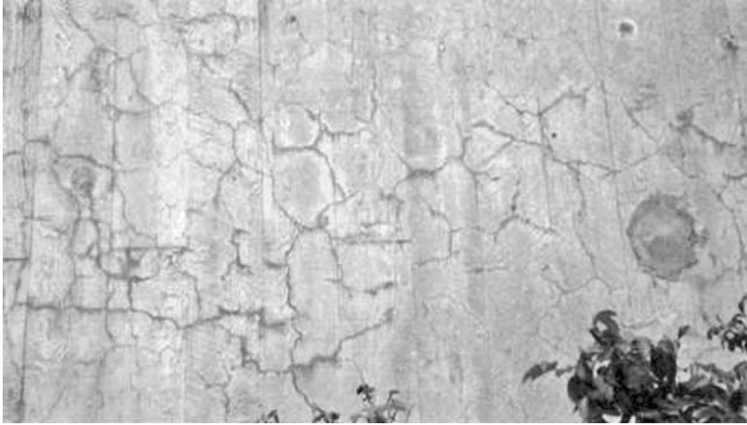
Fig. 4.8 Typical map cracking in a bridge abutment wing wall. Note that there is discoloration associated with some of the cracks
