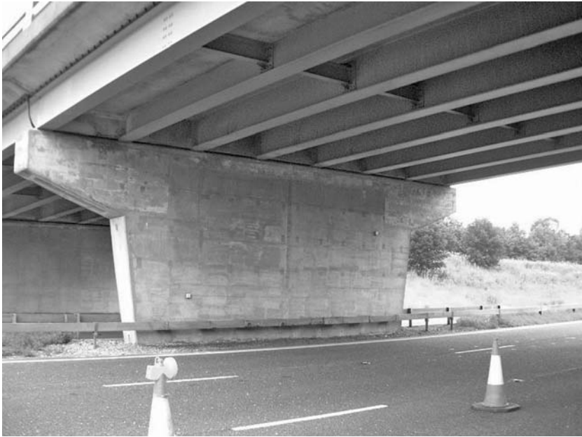
Fig. 11.12 Arc-sprayed zinc applied to a bridge on the M6 in Cumbria. The very top and the cantilevered ends of the leaf piers have probe anodes installed due to the higher moisture exposure
