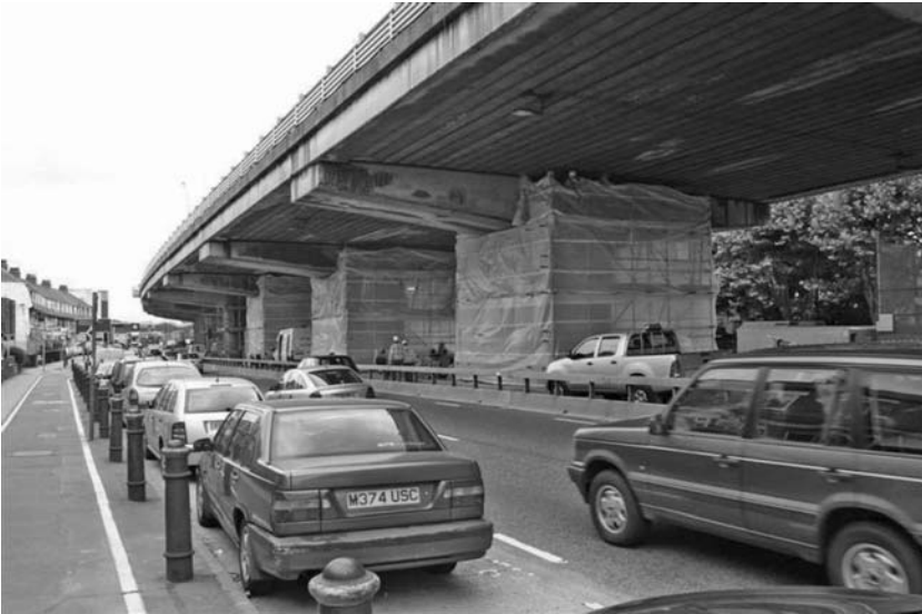
Fig. 10.34 Work had to be carried out safely without disruption to the traffic flow
