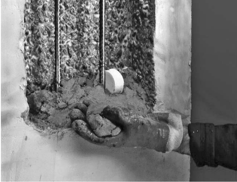
Fig. 11.16 A disk of zinc embedded in a proprietary mortar wired to the reinforcement exposed during repairs. (Reproduced with permission from Fosroc (UK) Ltd)
