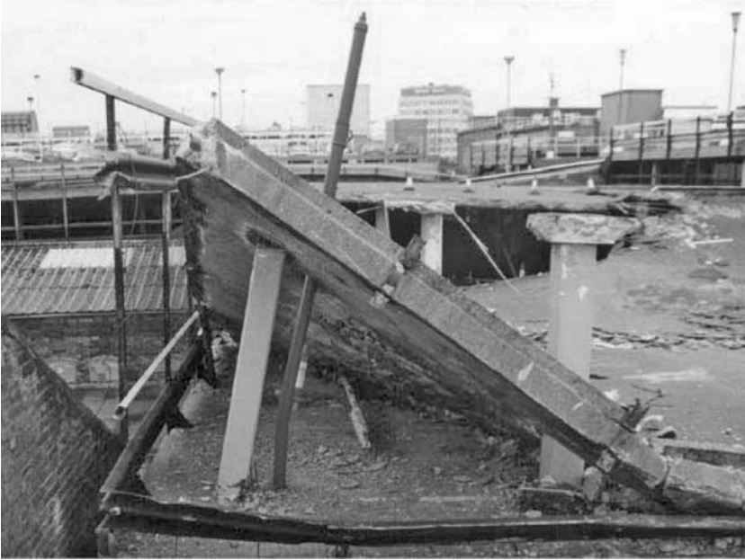
Fig. 1.6 The collapse of Pipers Row multi-storey car park in Wolverhampton
