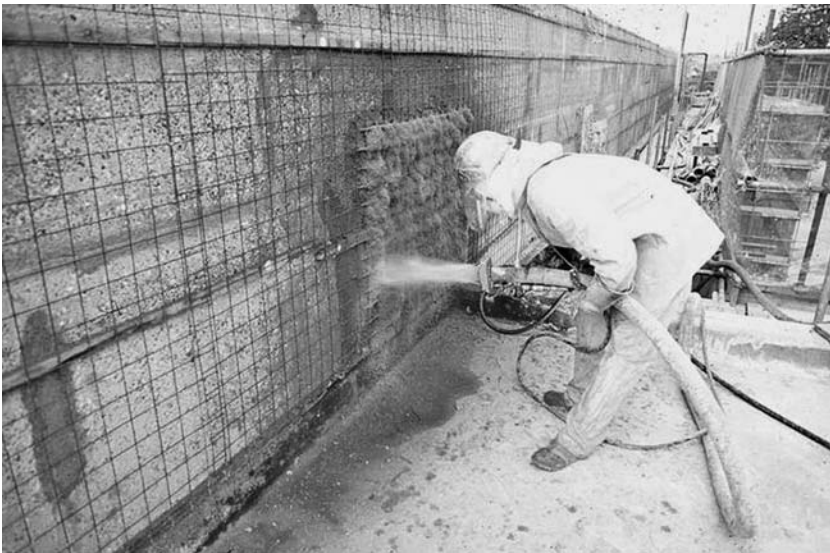
Fig. 11.18 Electrochemical chloride extraction steel mesh plus cellulose fibre overlay being applied. (Reproduced with permission from Makers Ltd)
