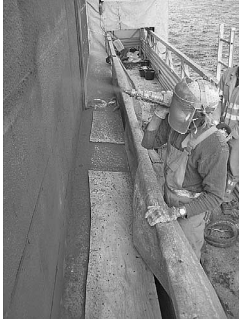
Fig. 11.11 Applying the conductive cementitious overlay to a bridge. (Courtesy of BASF – Construction Chemicals (UK) Ltd)
