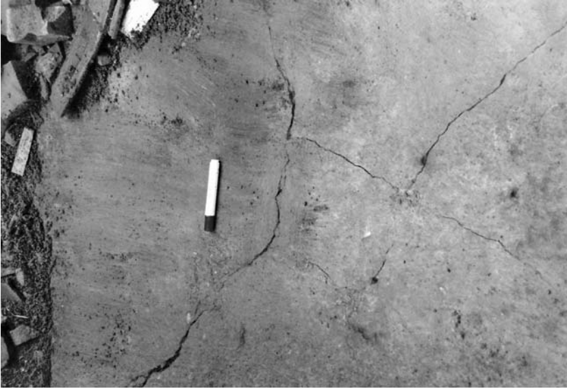
Fig. 4.4 Map pattern cracks due to external sulfate attacked in over-site concrete slab. (Courtesy of Ian Longworth)
