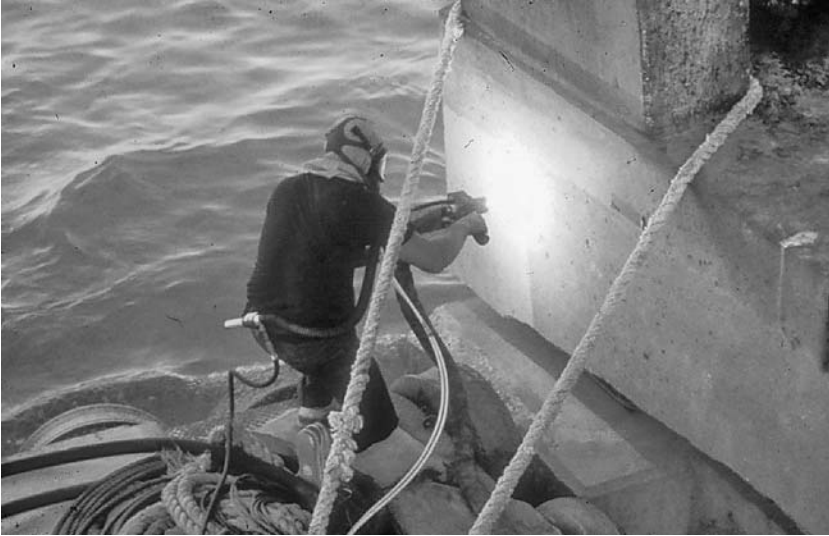
Fig. 11.13 Thermal spraying zinc on a bridge substructure in the Florida Keys. (Reproduced with permission from the Florida Department of Transportation)
