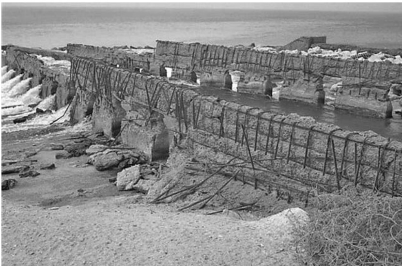
Fig. 3.3 Exfoliation of a seawall
