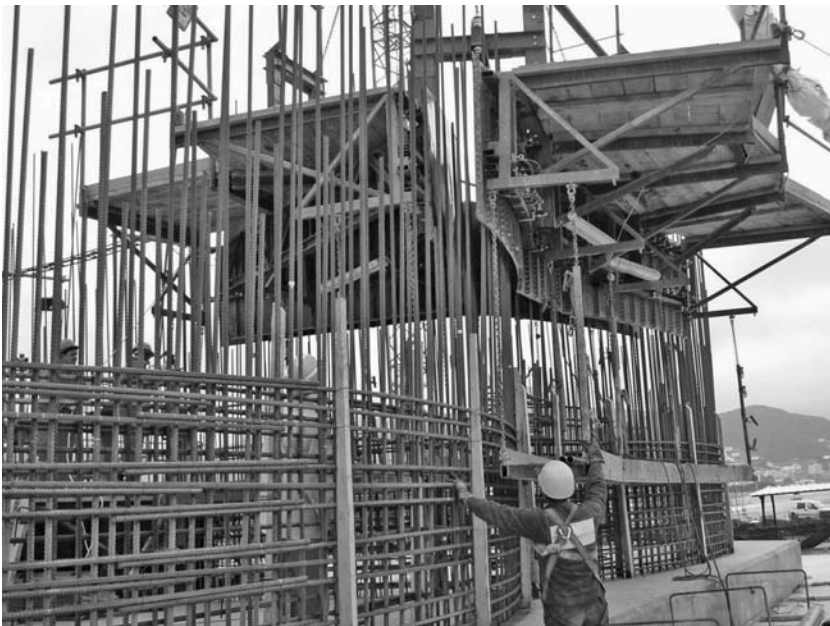
Fig. 10.18 Portion of the slipform being lowered into place for slipforming the walls
