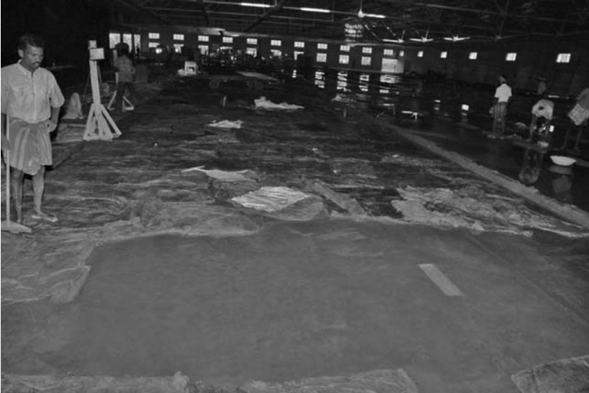
Fig. 10.47 Wet hessian curing. Ponding can also be seen in the top right of the picture
