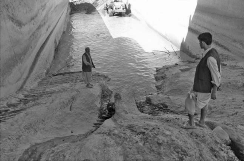
Fig. 3.2 Abrasion of concrete in a stilling basin
