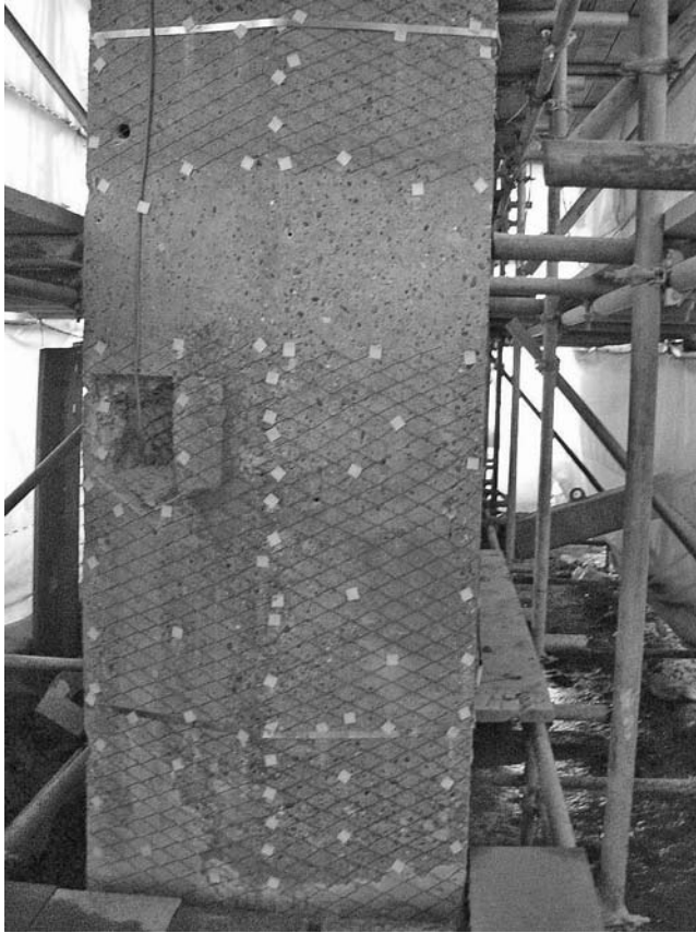
Fig. 11.8 A mixed-metal oxide-coated titanium mesh anode fixed to a concrete surface prior to applying a sprayed concrete overlay. (Courtesy of WS Atkins and the Highways Agency)
