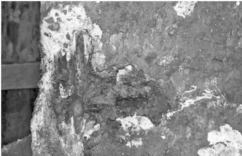
Fig. 10.26 Deep pitting corrosion to reinforcing bar in TSA-affected concrete
