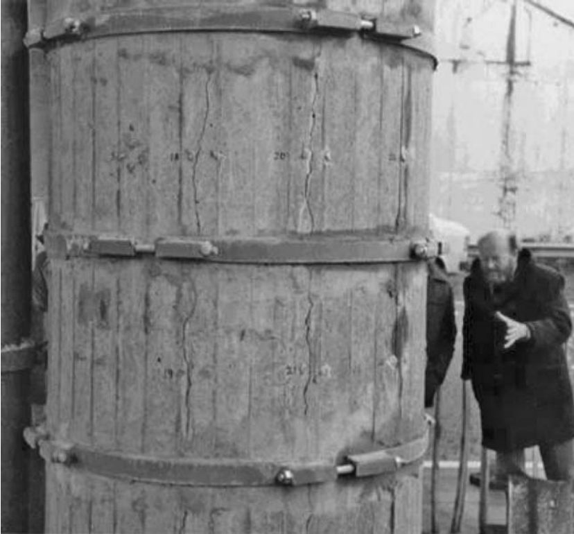
Fig. 4.9 A central bridge support column: note vertical cracks, the DEMEC monitoring points and the remedial measure of steel restraining hoops at 0.5 m centres
