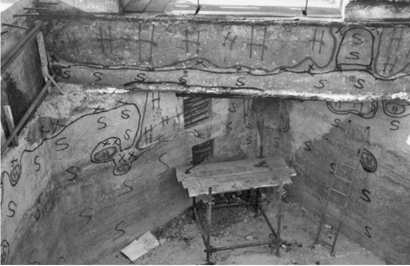
Fig. 10.5 Deterioration inside the caisson showing areas of hollowness (H)
