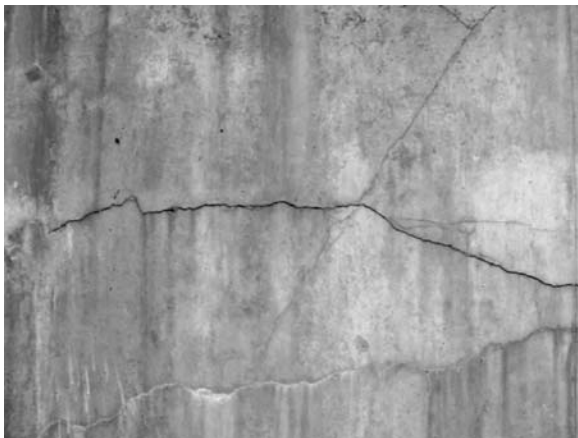
Fig. 10.10 Cracking to a crosshead
