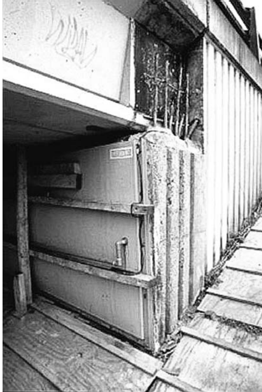
Fig. 11.19 Cassette-tank system using a mixed-metal oxide-coated titanium anode. (Reproduced with permission from Makers Ltd)
