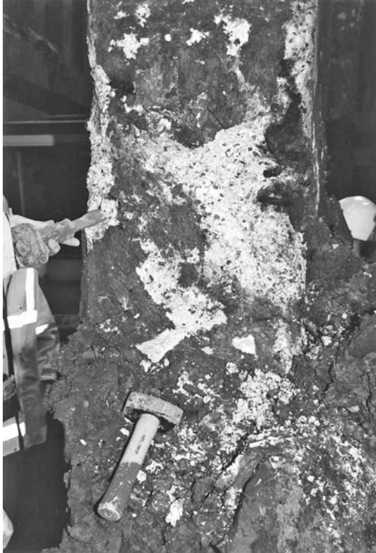
Fig. 4.2 Severe thaumasite form of sulfate attack at the base of a 29-year-old bridge column. (© 2003 Elsevier. Courtesy of Ian Longworth)
