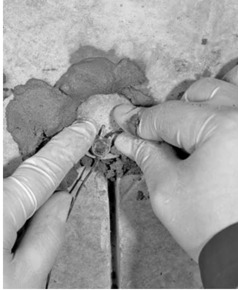
Fig. 11.17 A rod of zinc embedded in a proprietary mortar being inserted in a core hole in the concrete and connected in a string of other similar anodes to the steel to form an anode string or array. (Reproduced with permission from Fosroc 19 Ltd)
