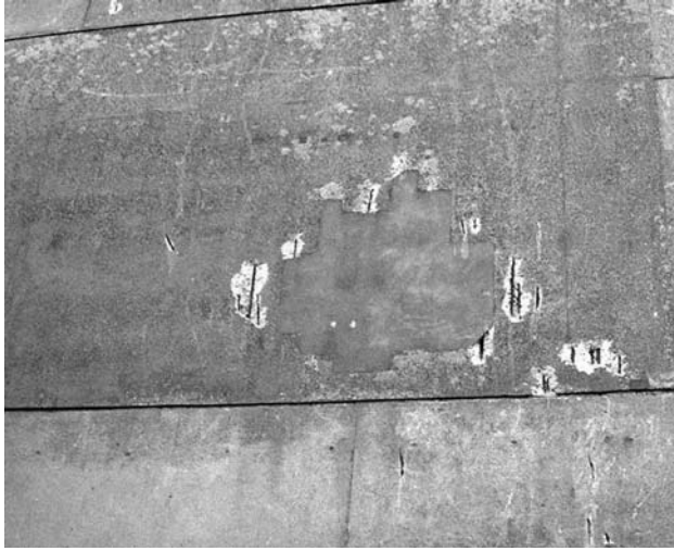
Fig. 11.4 A poorly executed patch repair with surrounding spalling due to incipient anodes on a building
