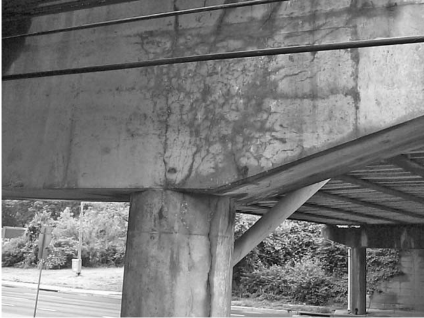
Fig. 4.3 Typical delayed ettringite formation associated damage in a precast concrete beam. (Reproduced by permission of the American Concrete Institute from Livingstone et al. 15 Courtesy of Richard Livingstone)
