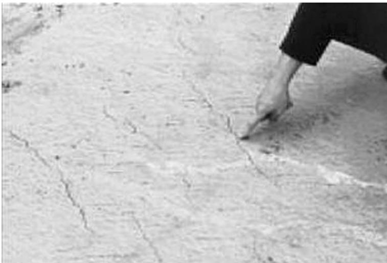
Fig. 7.10 Plastic cracking. (Courtesy of NRMCA)
