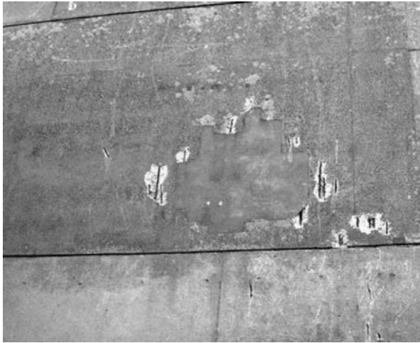
Fig. 10.40 Incipient anode formation around an old repair on the Biotower plant room prior to phase I repair and impressed current cathodic protection
