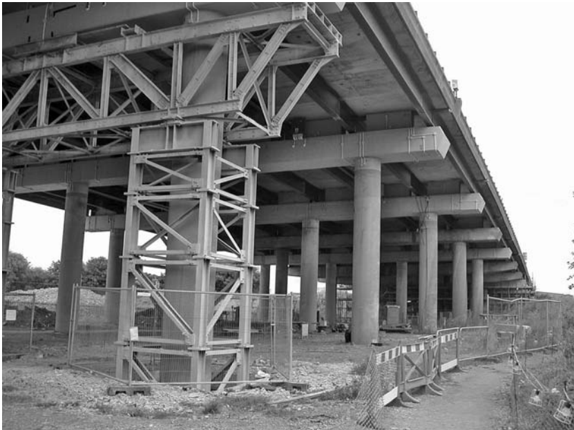
Fig. 11.1 Structural support system on the Midland Links Motorway elevated section (Junction 9, M6) prior to repair. The support system can be jacked up to take some of the load while concrete repair is undertaken. Conductive coating cathodic protection systems can be seen on cross heads in the background. (Courtesy of Kevin Davies, taken December 2005)
