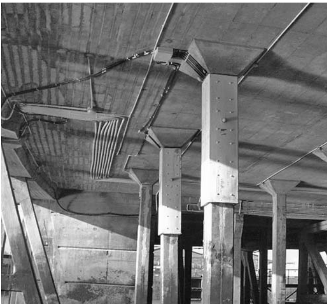
Fig. 11.15 Expanded zinc mesh anodes in a permanent form filled with cementitious grout and clamped to columns on a jetty in St Helier, Jersey
