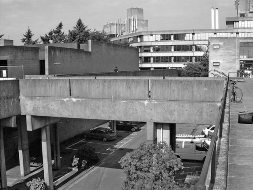
Fig. 10.39 Part of the library walkway showing the Teaching Wall and 'towers' behind. De-icing salts and leachate run-down can be seen where the waterproofing and drainage has failed, allowing corrosion of the slim pier supports
