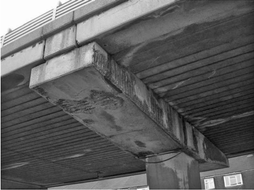
Fig. 10.31 Twin half joints contribute to the problems
