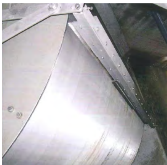
Figure 8.3 Rotary screen of the fine screen installation
