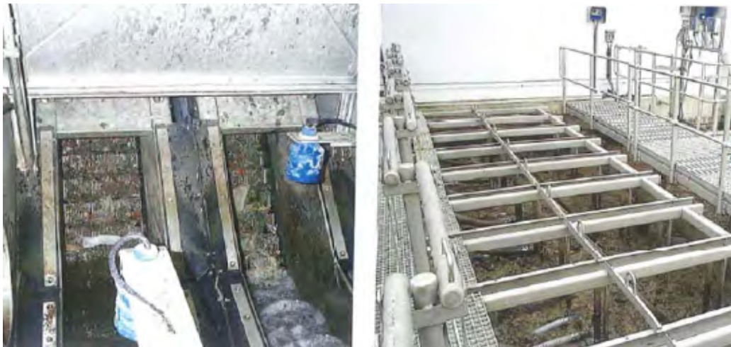
Figure 8.9 process stages at the Markranstadt wastewater treatment plant. Left: step screen, right: nitrification and de-nitrification tanks
