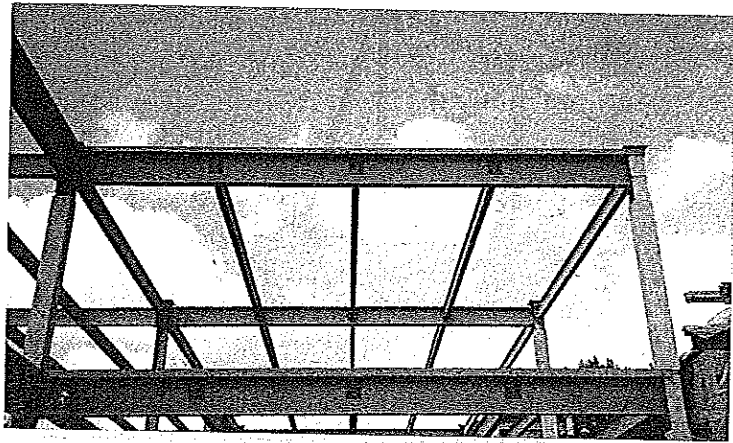
The simply supported beams and girders of this building frame were designed to resist the internal shear and moment acting throughout their lengths.
