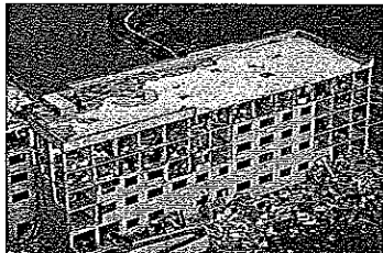
Hurricane winds caused this damage to a condominium in Miami, Florida.
