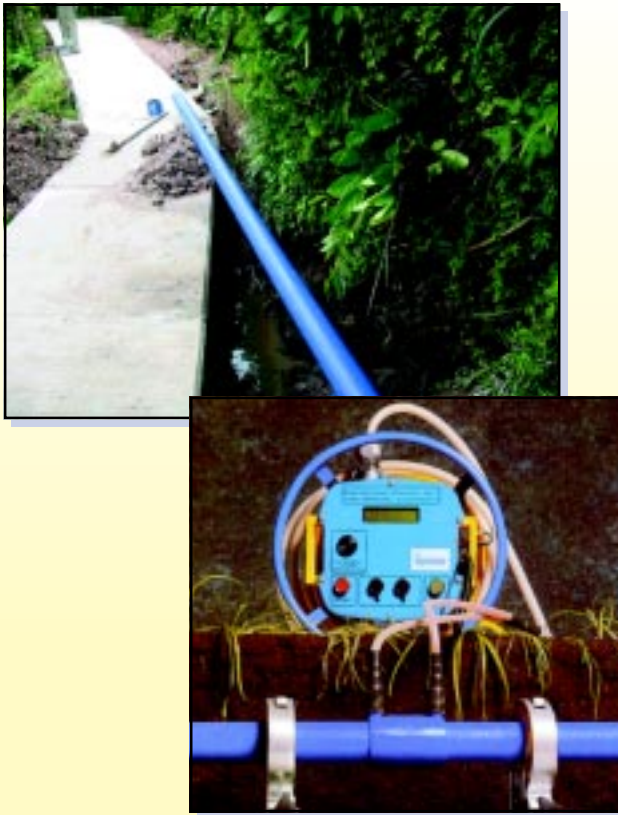
Figure 6 : Buried PE pipe along the most of the proposed alignment and Electrofusion Control Unit
