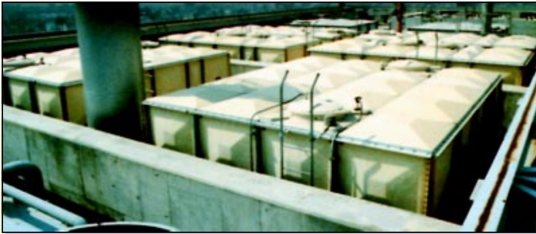
Figure 5 - GRP Tank with Brick Walls at Perimeter as Fire-break
