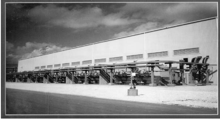
FIGURE 2.4.21 A 36-pulse system made up of 12 transformers with six types of six-pulse transformers for high-current electrochemical rectifier duty. Each transformer is 11,816-kVA OFWF with 426-V delta secondary windings. Each transformer has a 34,500-V primary with the shifts shown in Table 2.4.7 for a 36-pulse system. (Photo courtesy of Niagara Transformer Corp.)
