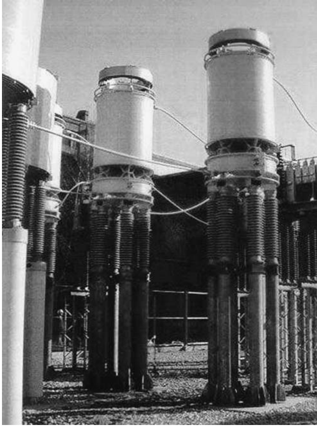
FIGURE 2.9.39 Tapped filter reactor with de-Q'ing rings.
