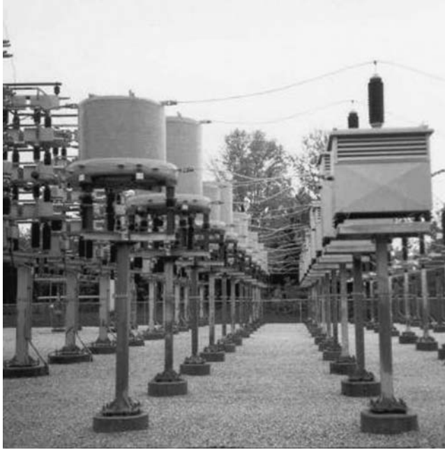
FIGURE 2.9.38 AC filter for an HVDC project; capacitors, tapped filter reactors, and separately mounted resistors.
