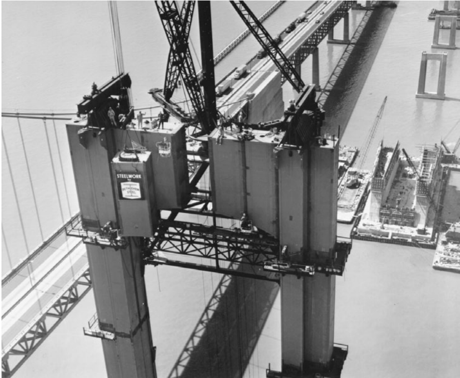
FIGURE 1.35 Tower erection, second Delaware Memorial Bridge, Wilmington, Del., 1966. Tower erection traveler has reached topmost erecting position and swings into place 23-ton closing top-strut section. Tower legs were jacked apart about 2 in. (50 mm) to provide entering clearance. Traveler jumping beams are in topmost working position, above cable saddles. Tower steelwork is about 418 ft (127 m) high. Cable anchorage pier is under construction at right. First Delaware Memorial Bridge (1951) is at left. The main span of both bridges is 2150 ft (655 m). (Courtesy of Bethlehem Steel Corporation.)
