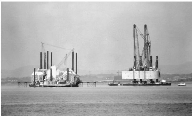
FIGURE 3.28 Installing precast concrete box caissons for Second Severn Crossing, Bristol, England. Extreme tidal range of 10 m and high tidal current imposed severe demands on installation procedures and equipment.
