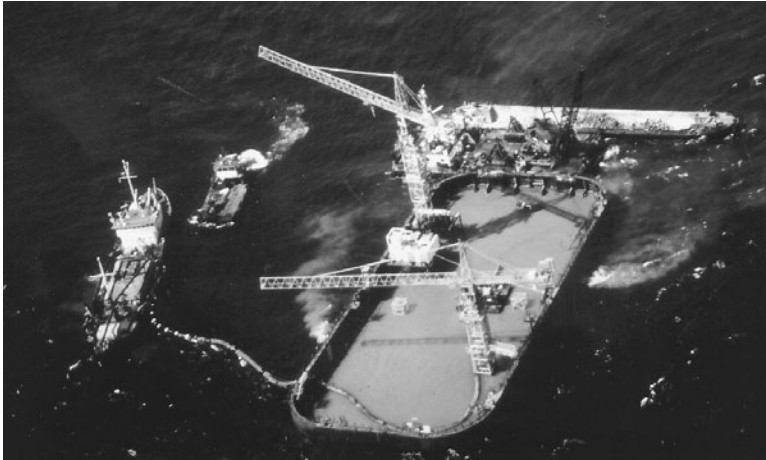
FIGURE 3.27 Prefabricated box caisson is floated into position, Great Belt Eastern Bridge, Denmark. Note temporary cofferdam above concrete caisson.
