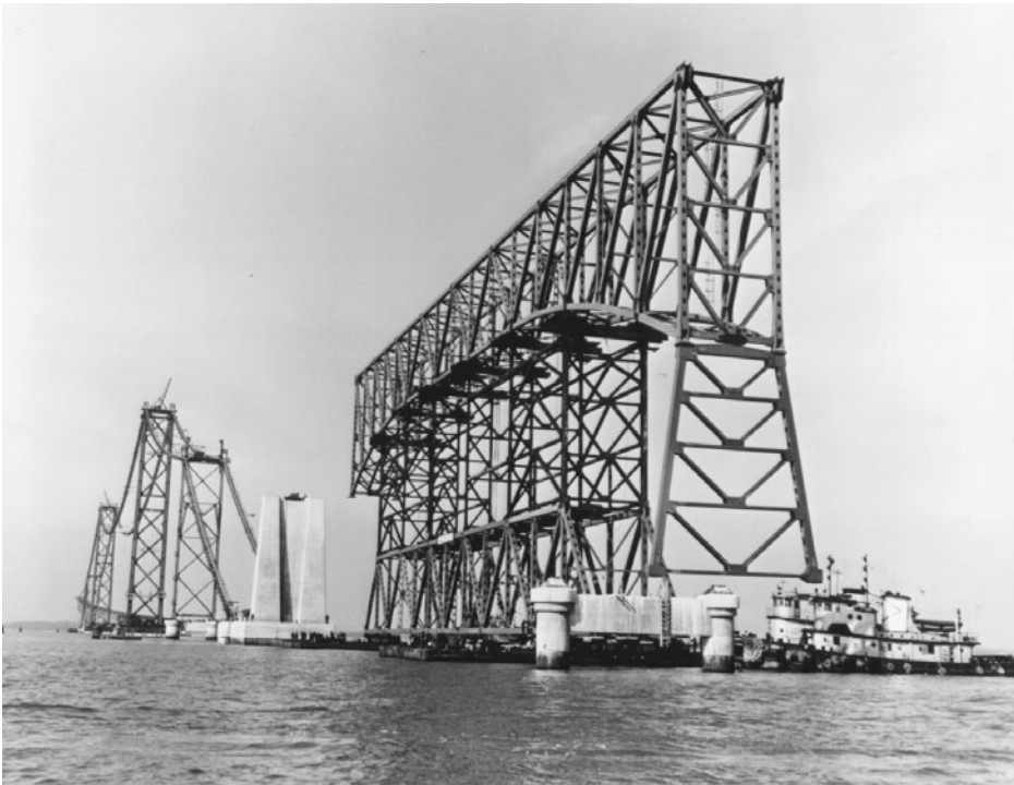
FIGURE 1.31 Floating-in erection of a truss span, first Chesapeake Bay Bridge, Maryland, 1952. A 480 ft (146 m) truss span, weighting 850 tons, supported on falsework consisting of a permanent deck-truss span along with temporary members, is being floated-in for landing onto its piers. Suspension bridge cables are under construction in background. (Courtesy of Bethlehem Steel Corporation.)
