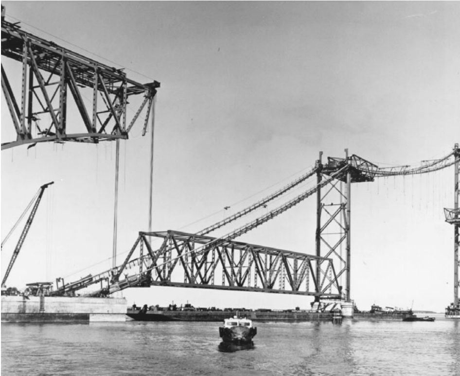
FIGURE 1.32 Erection of a truss span by hoisting, first Chesapeake Bay Bridge, Maryland, 1952. A 360 ft (110 m) truss span is floated into position on barges and picked clear using four sets of lifting falls. Suspension bridge deck is under construction at right. (Courtesy of Bethlehem Steel Corporation.)
