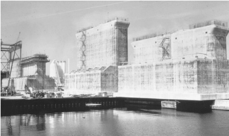
FIGURE 3.22 Prefabricated concrete box caissons are moved by jacks onto pier for load-out.
