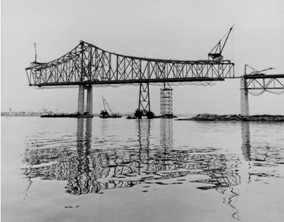
FIGURE 1.44 Closure of east side span, Commodore John Barry cantilever truss bridge, Chester, Pa., 1973. High-tower derrick boat (in background) started erection of trusses at both main piers, supported on falsework; then erected top-chord travelers for main and side spans. Sidespan traveler carried steelwork erection to closure, as shown, and falsework bent was then removed. East-mainspan traveler then cantilevered steelwork (without falsework) to midspan, concurrently with cantilever erection by west-half mainspan traveler, and trusses were closed at midspan. Commodore Barry has 1644 ft (501 m) main span, longest cantilever span in the U.S., and 822 ft (251 m) side spans. (Courtesy of Bethlehem Steel Corporation.)
