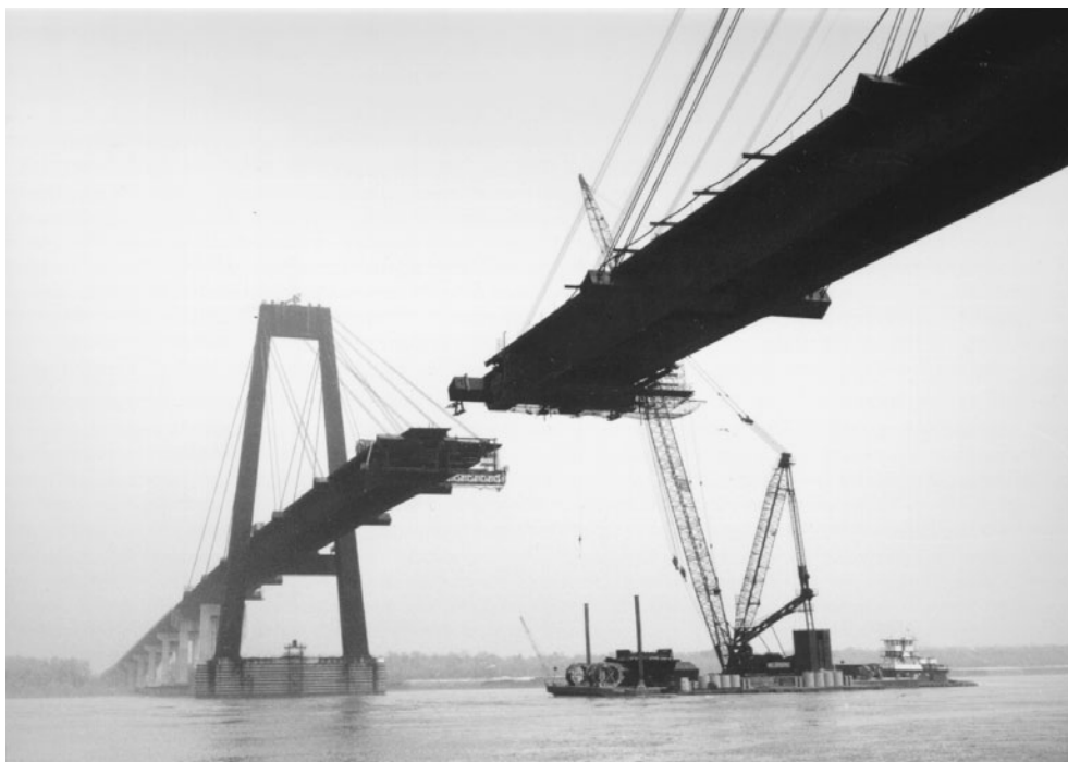
FIGURE 1.9 Cable-stayed orthotropic-steel-deck bridge over Mississippi River at Luling, La., 1982; view looking northeast. The main span is 1222 ft (372 m); the A-frame towers are 350 ft (107 m) high. A barge-mounted ringer derrick erected the main steelwork, using a 340 ft (104 m) boom with a 120 ft (37 m) jib to erect tower components weighing up to 183 tons, and using a shorter boom for deck components. Cable stays at the ends of projecting cross girders are permanent; others are temporary erection stays. Girder section 16-west of north portion of bridge, erected a few days previously, is projecting at left; companion girder section 16-east is on barge ready for erection (see Figure 1.10 ).
