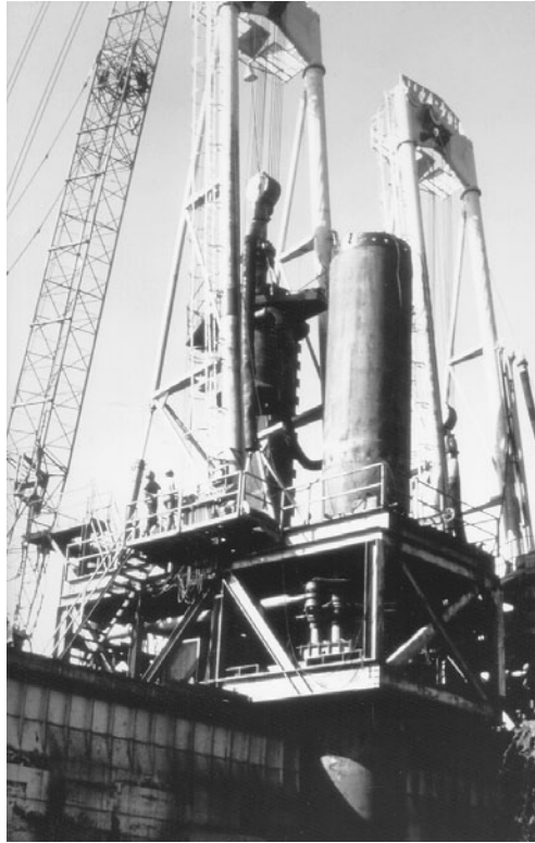
FIGURE 3.3 Steel tubular pile being installed from jack-up barge. Socket will be drilled into rock and entire pile filled with tremie concrete.
