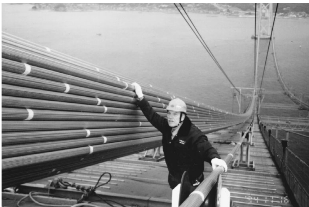
FIGURE 1.46 Parallel-wire-strand main cable, Akashi Kaikyo suspension bridge, Kobe, Japan, 1994. Main span is 6532 ft (1991 m), by far the world's longest. PWS at right is being towed across spans, supported on rollers. Completed cable is made up of 290 PWS, making a total of 36,830 wires, and has diameter of 44.2 in. (1122 mm) following compaction — largest bridge cables built to date. Each 127-wire PWS is about 2-3/8 in. (60 mm) in diameter. (Courtesy of Nippon Steel — Kobe Steel.)
