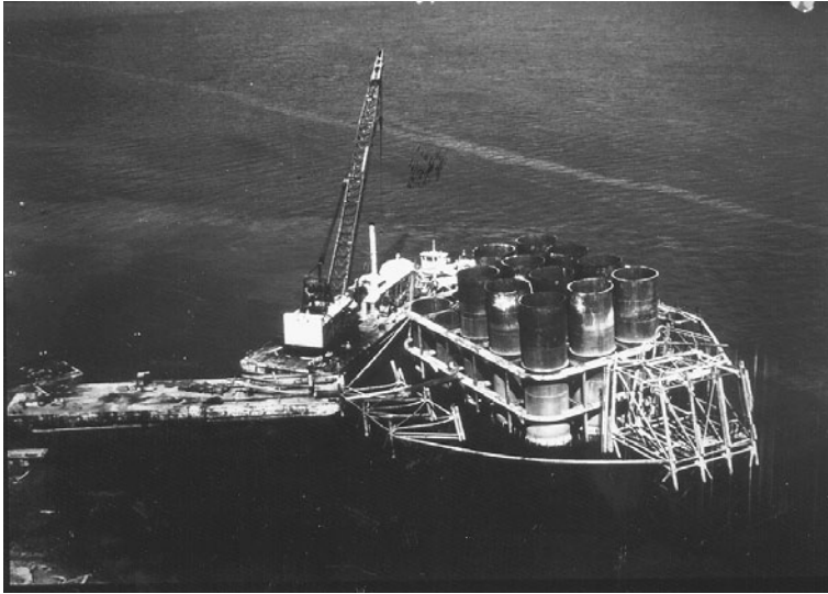
FIGURE 3.16 Open caisson for Sunshine Bridge across the Mississippi River. This caisson tipped during removal of false bottoms and is shown being righted by jacking against dolphins.
