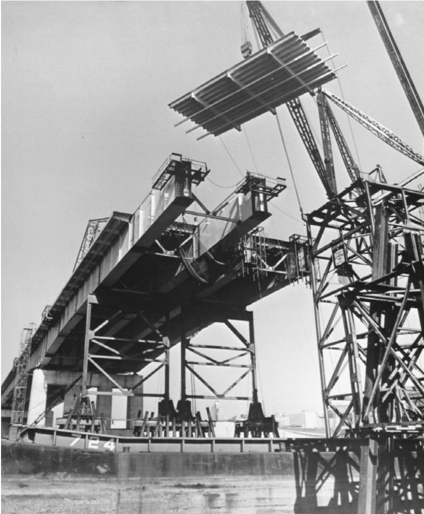
FIGURE 1.36 Erecting orthotropic-plate decking panel, Poplar Street Bridge, St. Louis, Mo., 1967. A five-span, 2165 ft (660 m) continuous box-girder bridge, main span 600 ft (183 m). Projecting box ribs are 5\frac{1}{2} \times 17 ft ( 1.7 \times 5.2 m) in cross-section, and decking section is 27 \times 50 ft ( 8.2 \times 15.2 m). Decking sections were field welded, while all other connections were field bolted. Box girders are cantilevered to falsework bents using overhead “positioning travelers” (triangular structure just visible above deck at left) for intermediate support. (Courtesy of Bethlehem Steel Corporation.)
