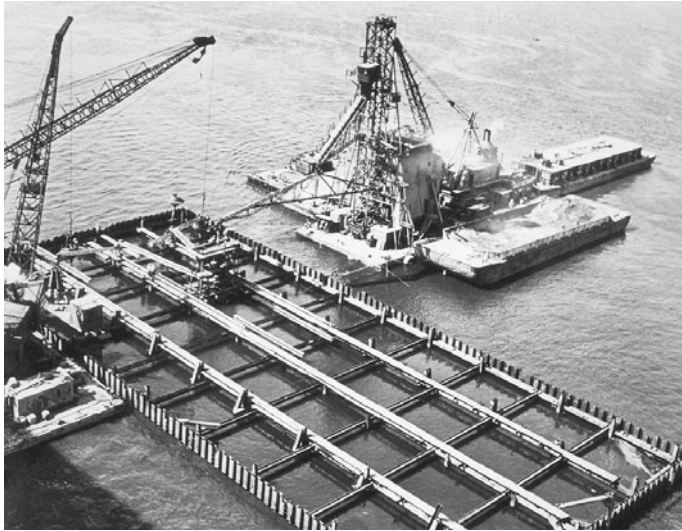
FIGURE 3.9 Large steel sheet pile cofferdam for Second Delaware Memorial Bridge, showing bracing frames.
