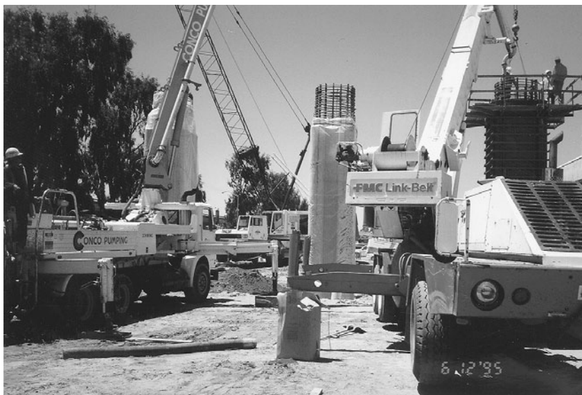
FIGURE 4.2 Crane used to hold the column cage; column is being cured with plastic wrap.
