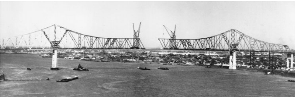
FIGURE 1.34 Greater New Orleans cantilever bridge, Louisiana, 1957. Tall double-boom deck travelers started at ends of main bridge and erected anchor spans on falsework, then the 1575 ft (480 m) main span by cantilevering to midspan. (Courtesy of Bethlehem Steel Corporation.)
