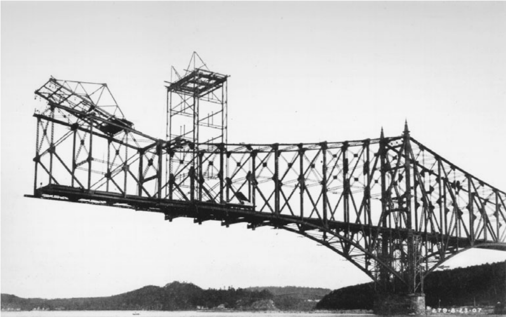
FIGURE 1.11 First Quebec railway cantilever bridge, 23 August 1907. Cantilever erection of south main span is shown six days before collapse. The tower traveler erected the anchor span (on falsework) and then the cantilever arm; then erected the top-chord traveler, which is shown erecting suspended span at end of cantilever arm. The main span of 1800 ft (549 m) was the world's longest of any type. The sidespan bottom chords second from pier (arrow) failed in compression because latticing connecting chord corner angles was deficient under secondary bending conditions.
