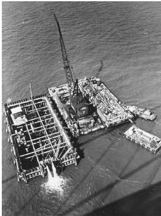
FIGURE 3.12 Dewatering the cofferdam for the main tower pier, Second Delaware Memorial Bridge.
