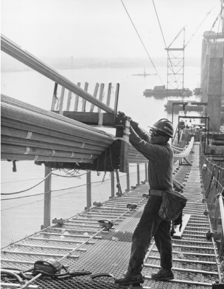
FIGURE 1.37B Cable formers maintain strand alignment in cables prior to cable compaction. Each finished cable is about 15-1/4 in. (387 mm) in diameter. (Courtesy of Bethlehem Steel Corporation.)
