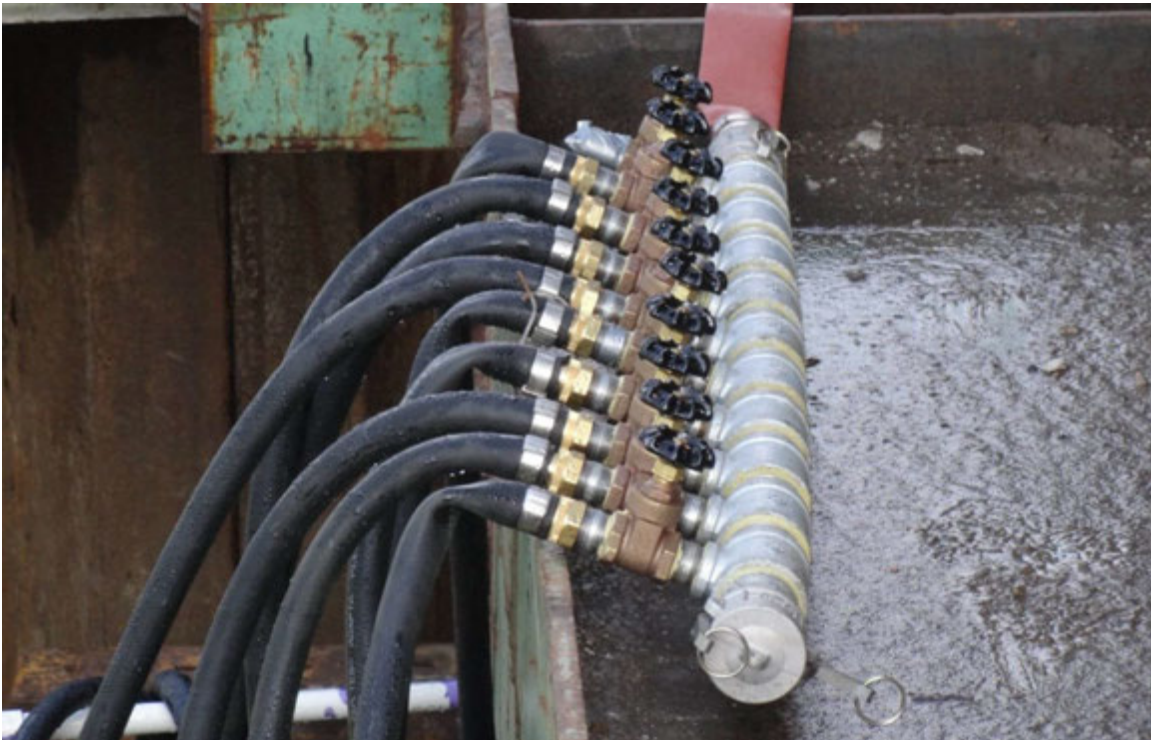
Figure 5.18 US 34 Bridge cooling pipe system manifold
