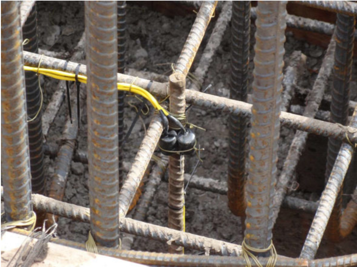
Figure 2.12 Installed thermal monitoring sensor
