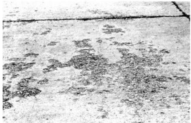
Fig. 11.5—Scaling is the loss of surface mortar, usually exposing the coarse aggregate
