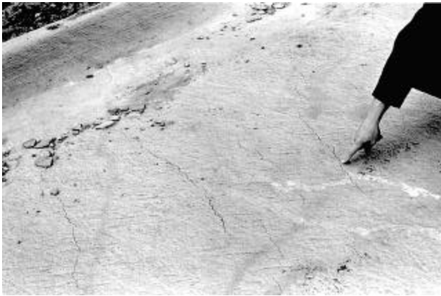
Fig. 11.2.2.1—Plastic shrinkage cracks are caused by rapid loss of mix water from the surface while the concrete is still plastic
