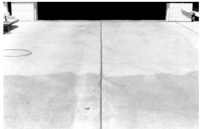
Fig. 11.9—Concrete slab discoloration due to the use of calcium chloride admixture. Concrete in the upper part of the photo did not contain the admixture
