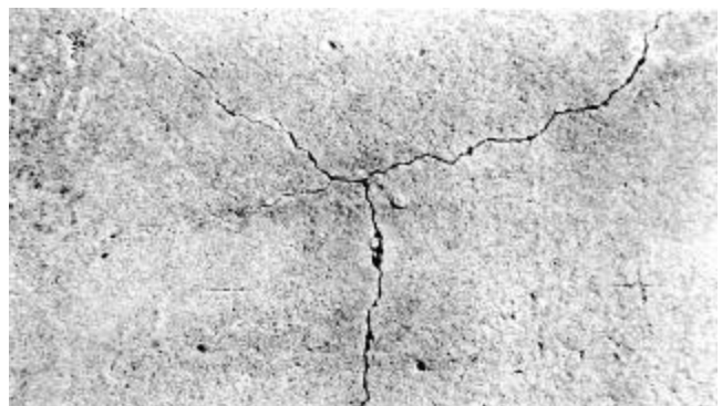
Fig. 11.2—Drying shrinkage cracks such as these are a frequent cause of complaint
