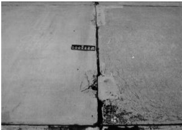
Figure 5.8. Point bearing causing failure
