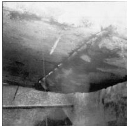
Figure 4.2. Bottom of deteriorated slab
