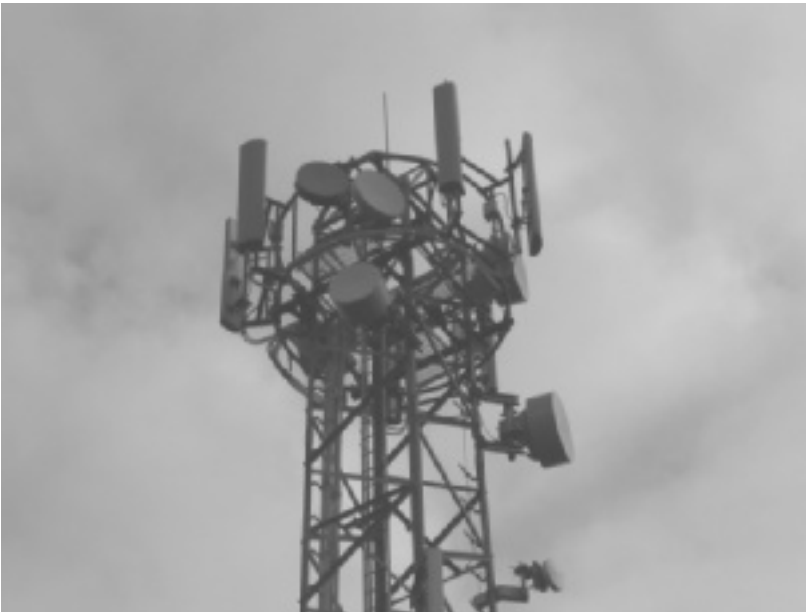
Figure 5.57 Installed antennas and supporting structure
