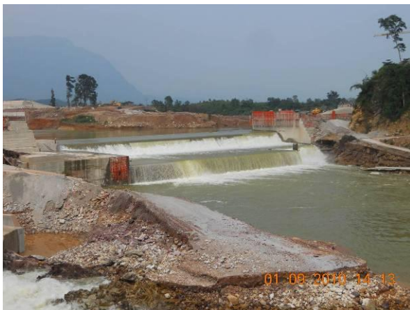
Figure 8 RCC spillway being overtopped after first flood
