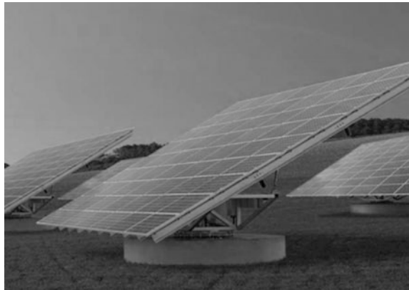
Fig. 7.6 Azimuth one axis tracking system
