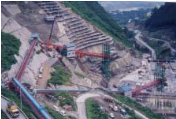
Figure 21. Belt Conveyor from Aggregate Production Plant to Dam Site
