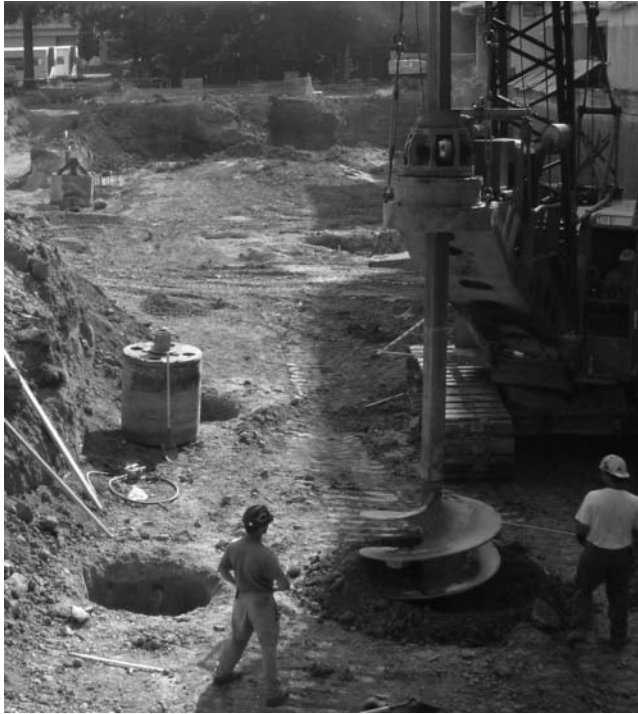
Figure 12.5 Drilled shaft construction using the dry method (Courtesy of Sanjeev Kumar, Southern Illinois University, Carbondale, Illinois)
