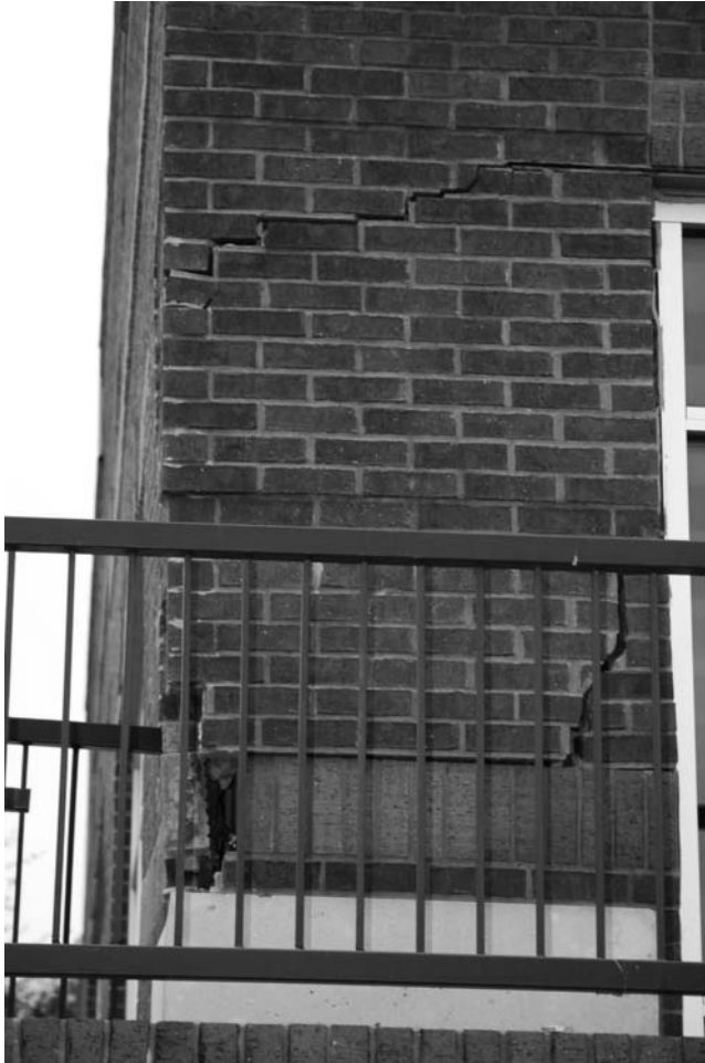
Figure 13.8 Cracks in a wall due to heaving of an expansive clay (Courtesy of Anand Puppala, University of Texas at Arlington, Arlington, Texas)
