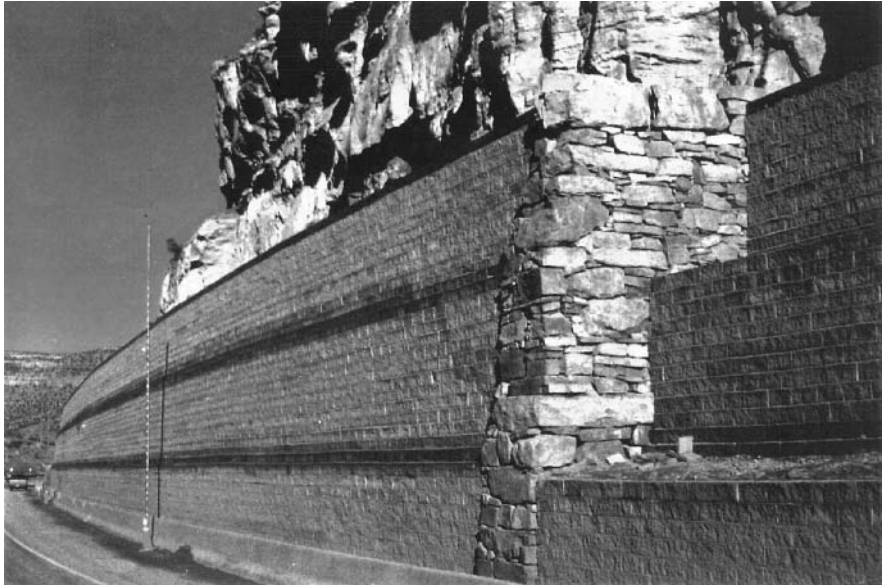
Figure 8.35 A completed geotextile-reinforced retaining wall in DeBeque Canyon, Colorado (Courtesy of Jonathan T. H. Wu, University of Colorado at Denver, Denver, Colorado)
