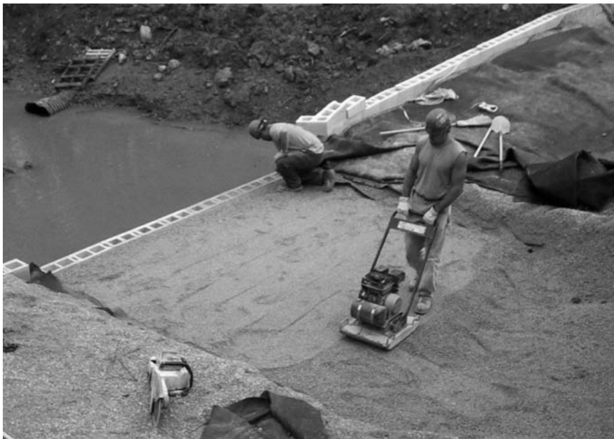
Figure 8.34 Construction of a geotextile-reinforced retaining wall (Courtesy of Jonathan T. H. Wu, University of Colorado at Denver, Denver, Colorado)
